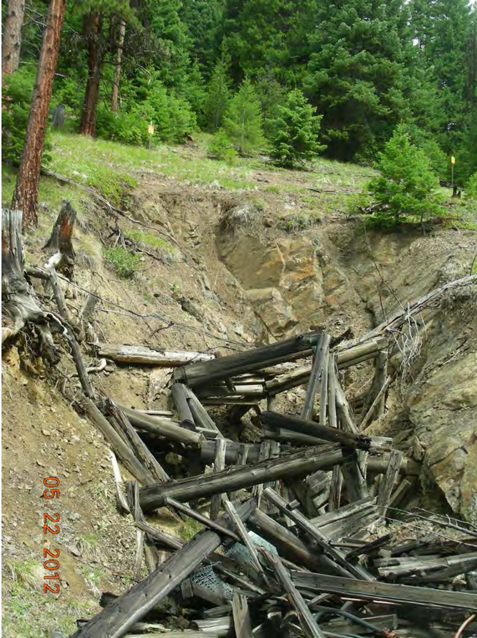
New Independence Crosscut, note FS property is behind signs above collapsed portal
