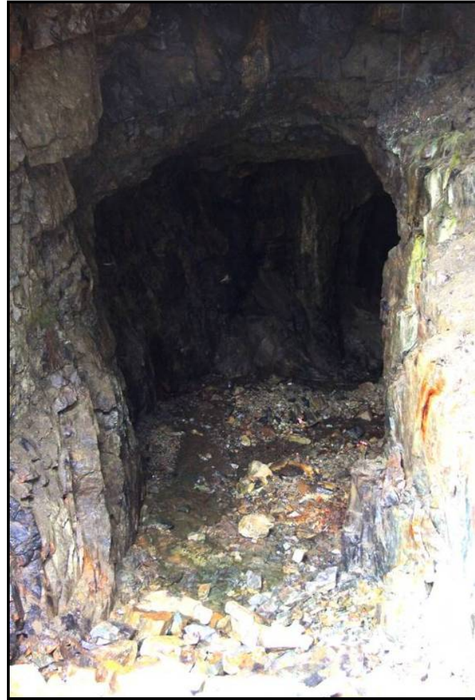
Figure 2-12. Photograph Looking South in the 900-Foot Level Portal, showing water flowing from the rock pile which partially blocks the portal. (The photo also shows the adit bending toward the right (west) approximately 100 feet inside the portal.)
