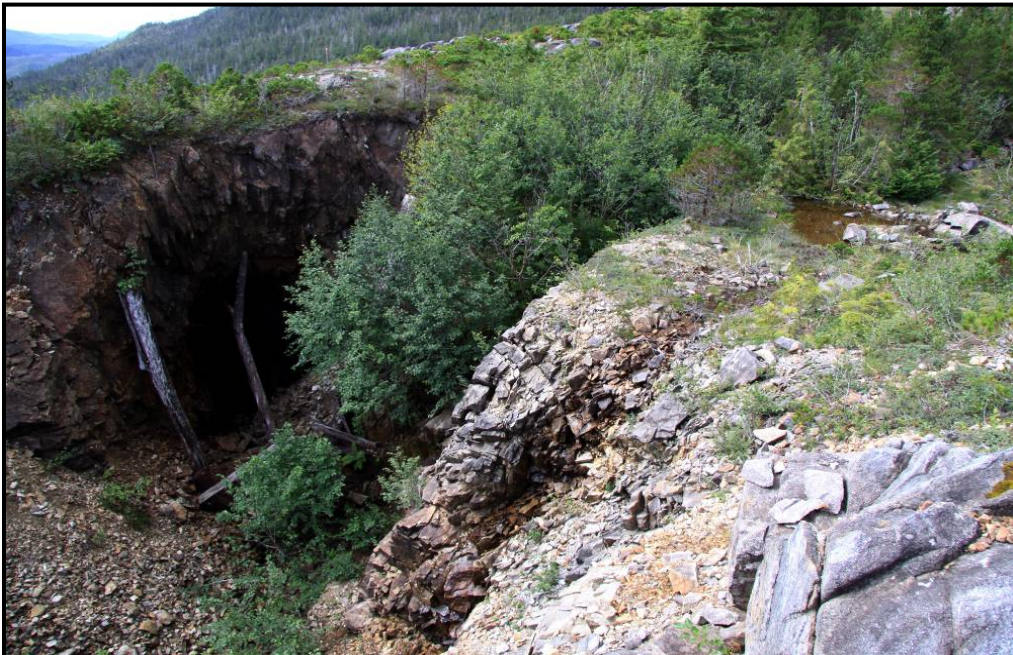
Figure 2-9. Photograph Looking Southwest Down into the Open Pit and 900-Foot Level portal showing the point at which surface runoff from the north and west (seen on the right side) enters the pit.
