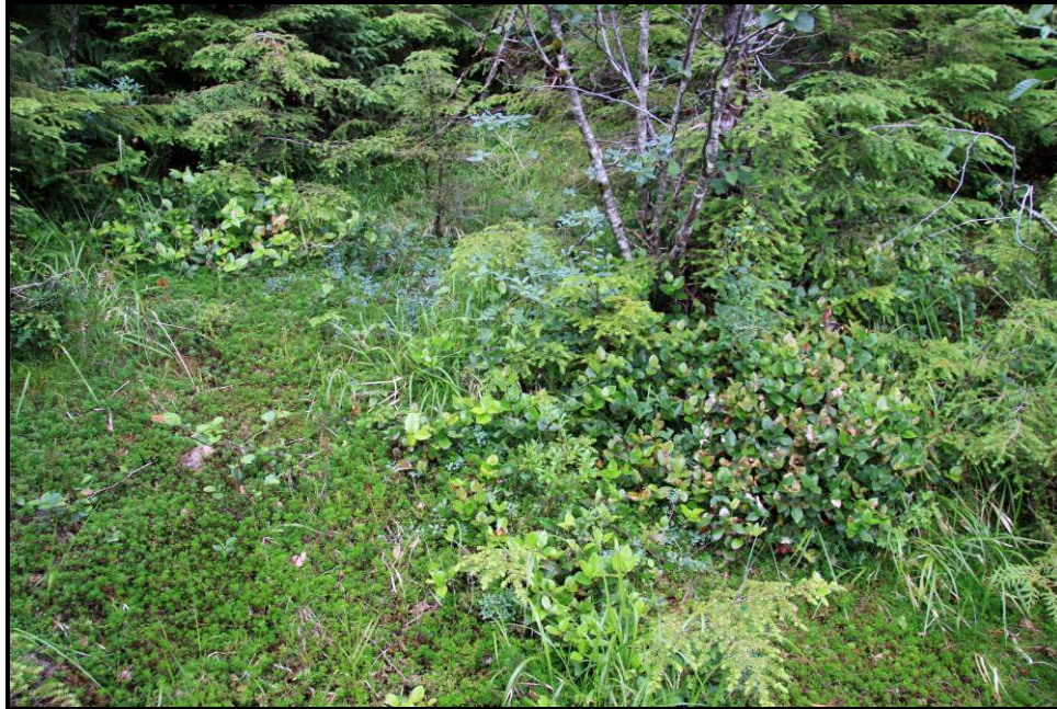
Figure 4-15. Photo looking north at the downstream face of the dike, illustrating the type and species of vegetation which have developed over the surface
