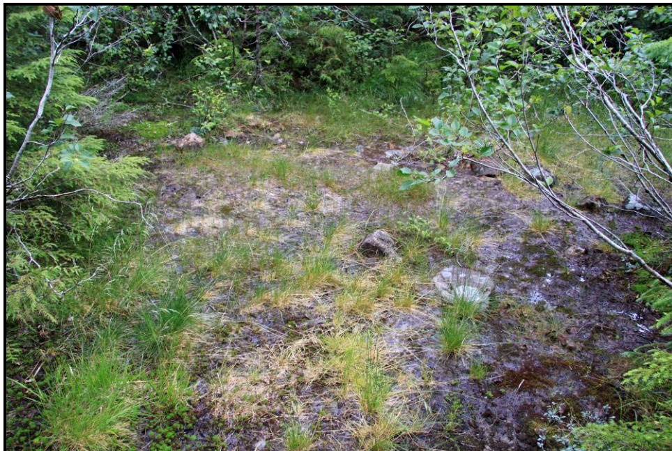
Figure 4-16. Photo looking north at the seepage coming from the downstream (south) toe of the Open Pit dike
