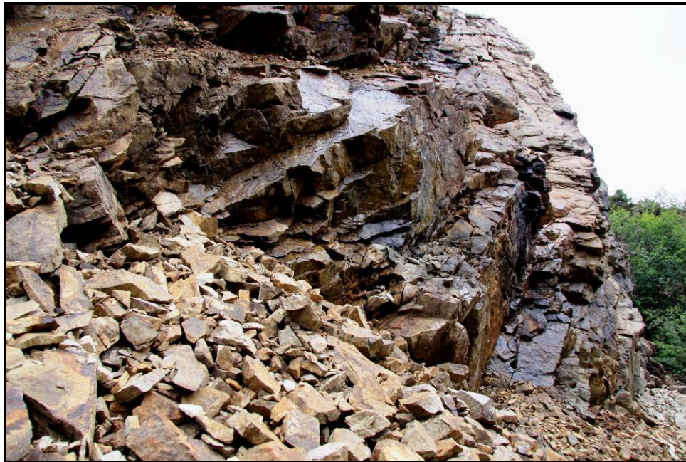
Figure 4-13. Photo looking north on the west wall of the Open Pit, showing groundwater seepage from bedrock fractures (The wall was dry for approximately 10 feet below the rim).
