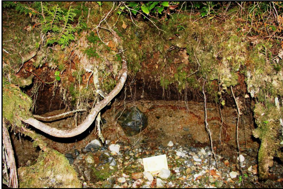
Figure 4-41. Photo showing the soil profile in the road cut immediately above the east landslide, illustrating the distinct soil types and saturation of the local soils
