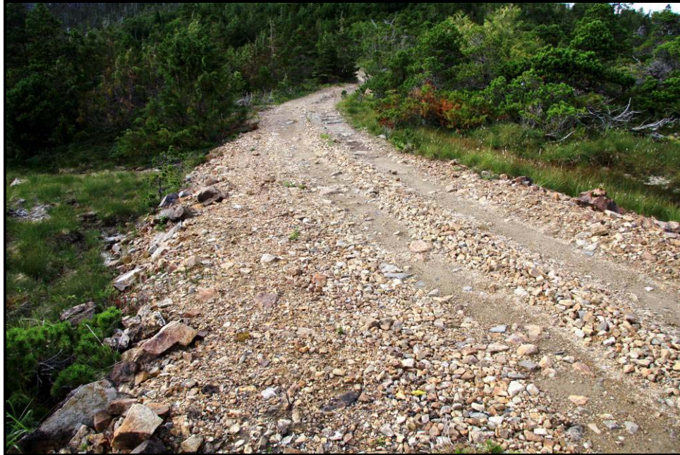
Figure 4-37. Photo looking north at the I&L access road taken from just north of the 900-Foot Level haul road
