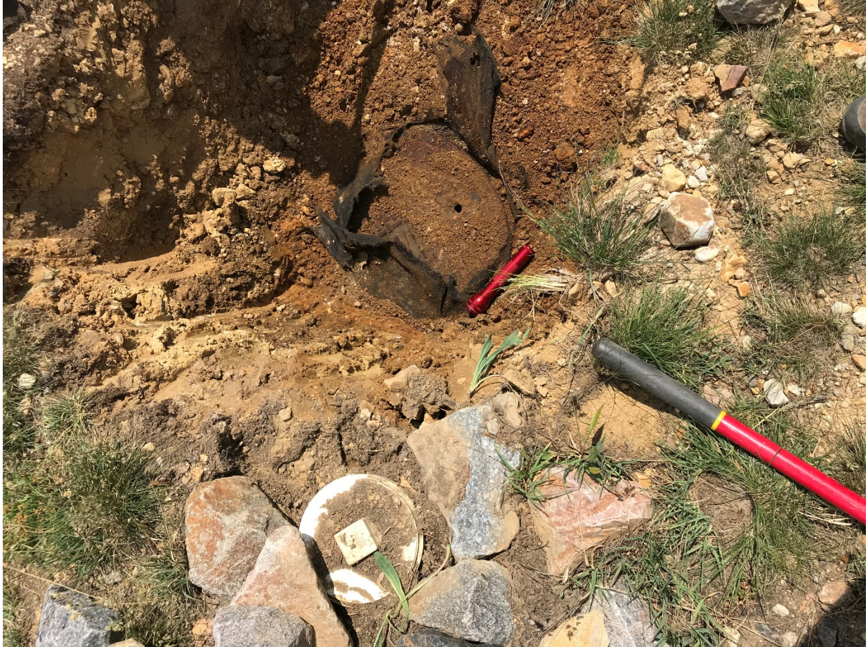
Photo 1. View of McLaren Adit drain access manhole and PVC cleanout pipe from above. Manhole is west (downhill) of PVC cleanout and approximately 36 inches below ground surface.
