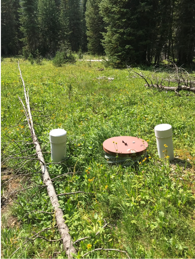
Eastern valve box
