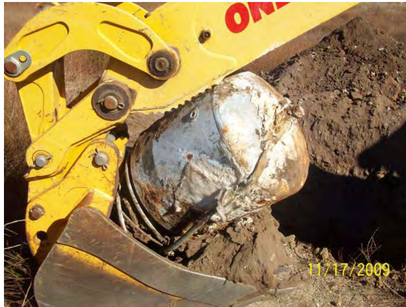
Photograph A-7. Subsurface metal debris, suspected water heater (PH-2).
