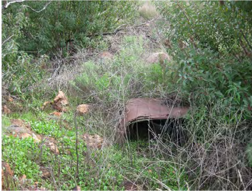
Photograph A-15. Metal surface debris (roof of car) exposed in drainage east of burn dump site.
