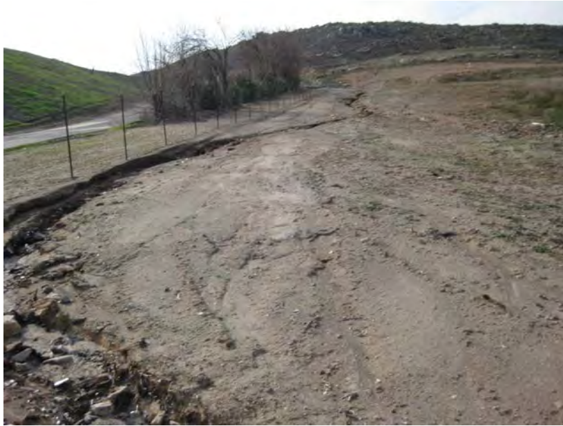
Photograph A-11. Newly eroded gully observed during second site visit along southern edge of site (in area recently hydroseeded by Allied Waste); facing west.
