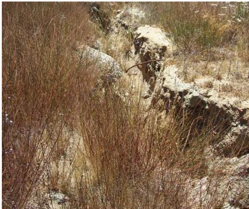
Photograph A-4. Drainage channel erosion along northeastern edge of site.
