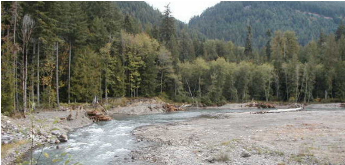
Figure 1- Engineered log jams along the mainstem Cispus River just upstream of Road 28 bridge (Tom Music Bridge) completed in Fall, 2001.
