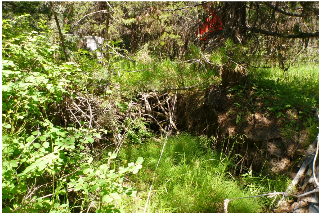
Figure 12. Headcut moving through decommissioned roadbed because of plugged culvert (current stream channel over roadbed).
