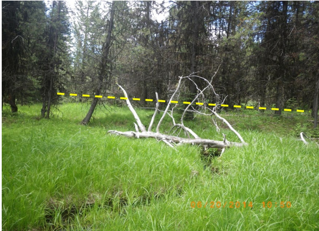
Figure 11. Decommissioned road crossing that needs to be removed from the Tinker Creek floodplain. Yellow dashed line highlights the old roadbed crossing the valley floor. The plugged culvert (complete fish passage barrier) and sediment delta are beyond the roadbed in the picture.
