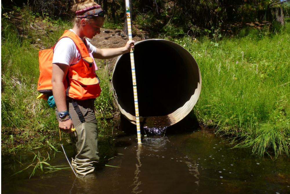
Figure 3. National Forest System Road 3620000 aquatic organism passage culvert replacement (looking upstream) that will be completed under a 2019 Aquatic Restoration Decision checklist
