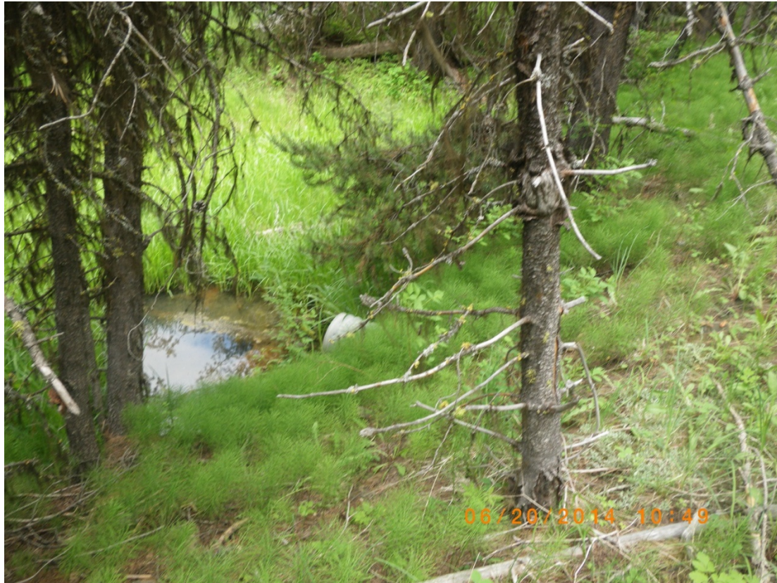
Figure 13. Decommissioned roadbed with undersized culvert still in place (downstream side).
