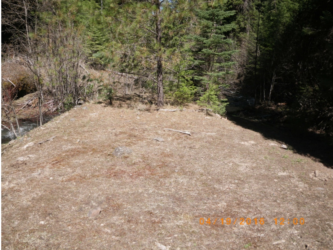
Figure 7. Butte Creek at National Forest System Road 2050072 showing road fill on floodplain
