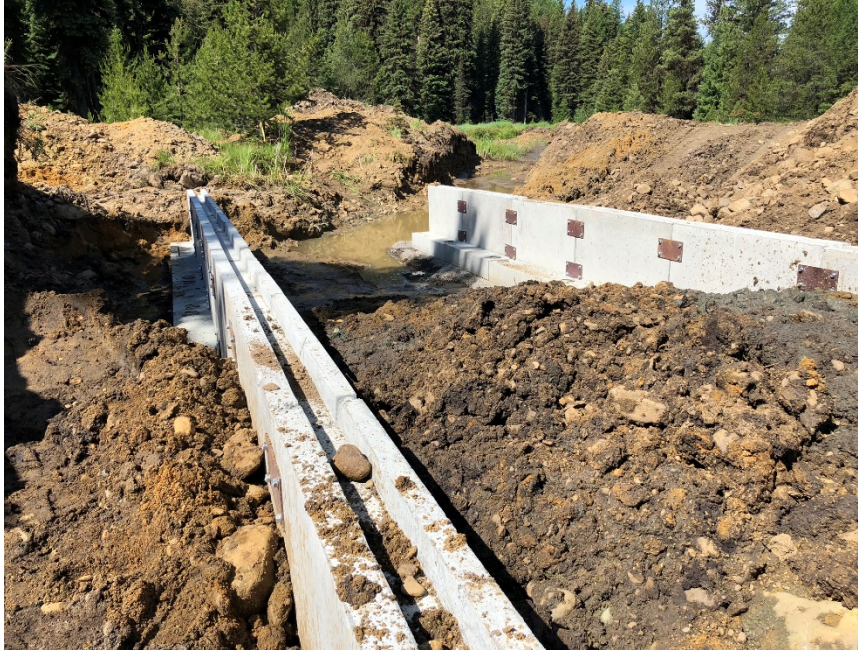
Figure 29. Example of what aquatic organism passage culvert construction can look like (footer placement on Big Creek in 2018)
