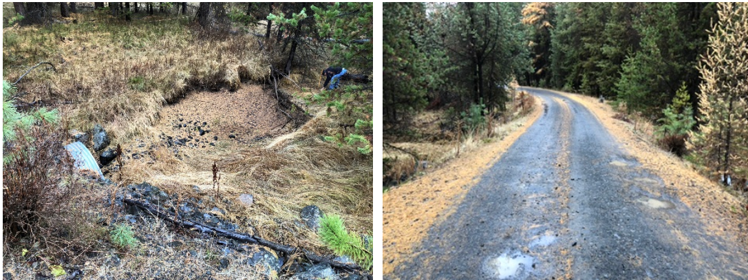
Figure 18. National Forest System Road 2622 culvert on Summit Creek and a view of the road
