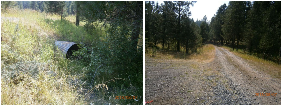
Figure 13. National Forest System Road 1940 culvert on Summit Creek (culvert inlet and the road the culvert is on)
