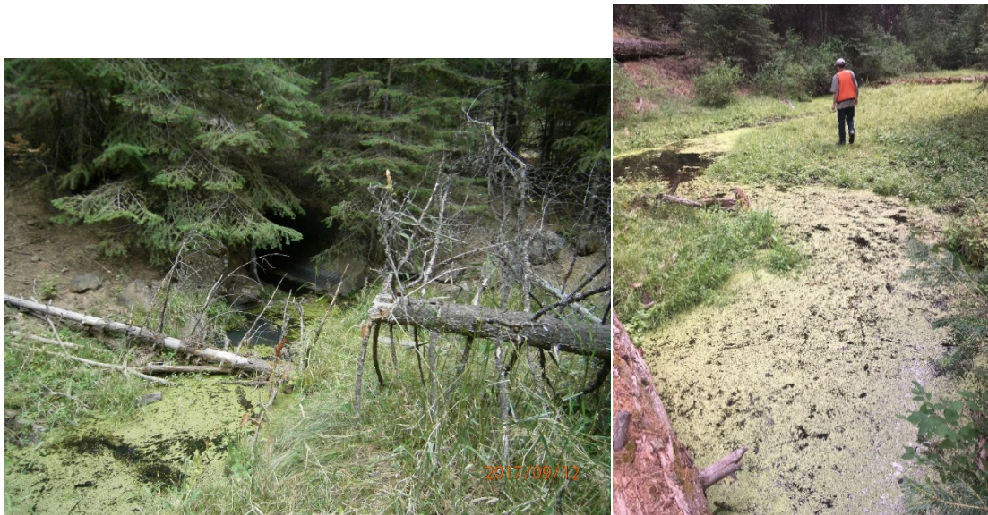
Figure 26. East Fork Deer Creek National Forest System Road 4020 culvert Inlet and directly upstream of the inlet (gradient change upstream and downstream of culvert is evident)
