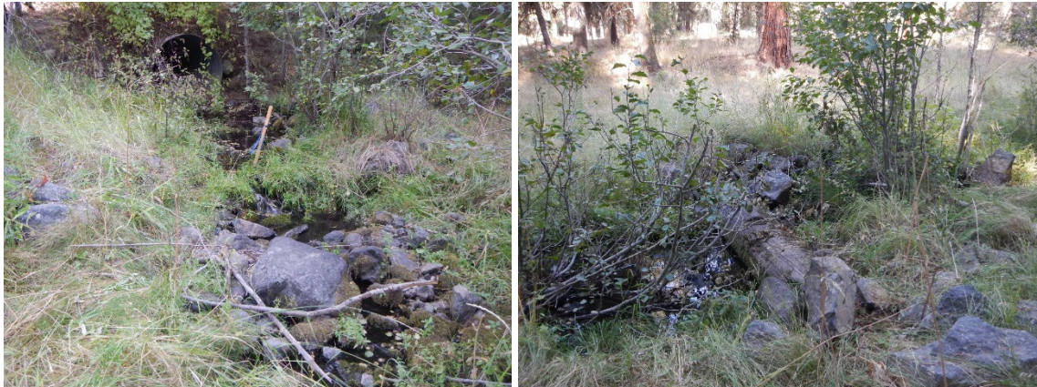
Figure 21. National Forest System Road 2622172 culvert on Idaho Creek and log weir downstream in channel near culvert
