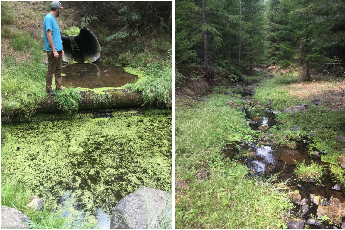
Figure 25. East Fork Deer Creek National Forest System Road 4020 culvert outlet and downstream of the outlet farther from the influence of the culvert
