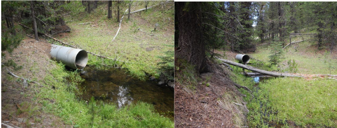
Figure 5. Existing Tinker Creek culvert outlet, perched and undersized
