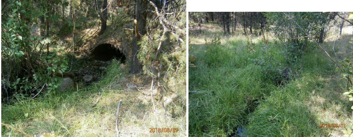
Figure 15. National Forest System Road 1940281 culvert on Summit Creek and general creek area
