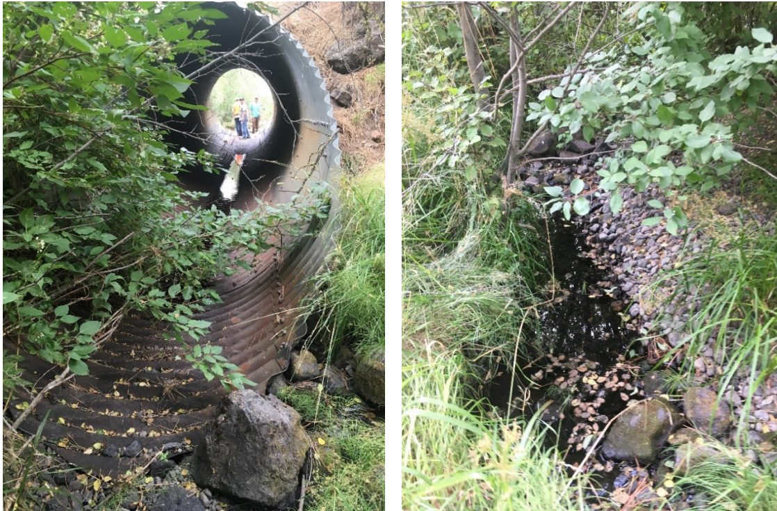
Figure 2. National Forest System Road 3600052 East Fork Beech Creek culvert inlet and upstream of the inlet
