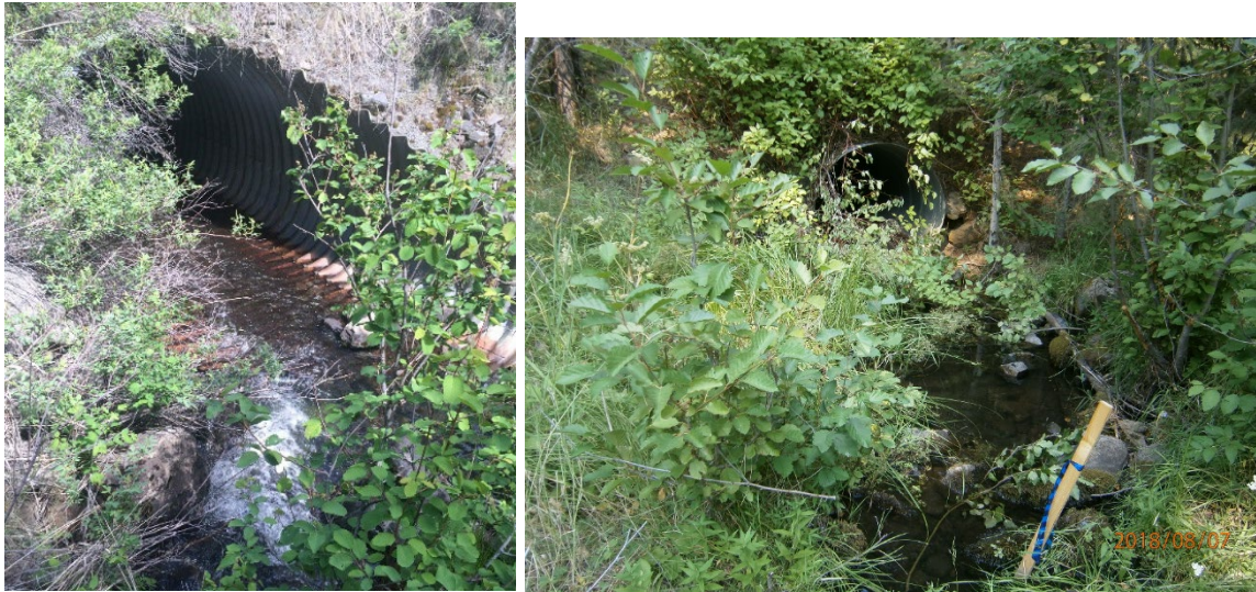
Figure 7. National Forest System Road 36 culvert on Cottonwood Creek (left photo: inlet, right photo: outlet)
