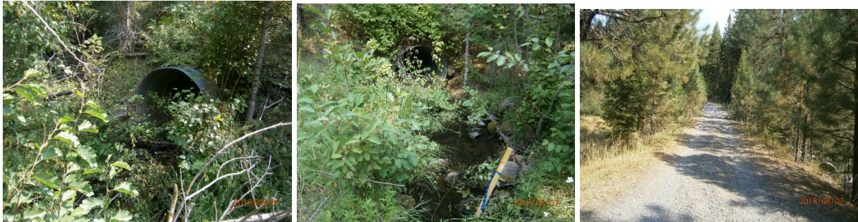
Figure 22. National Forest System Road 262172 culvert on Idaho Creek and road that culvert is being replaced on
