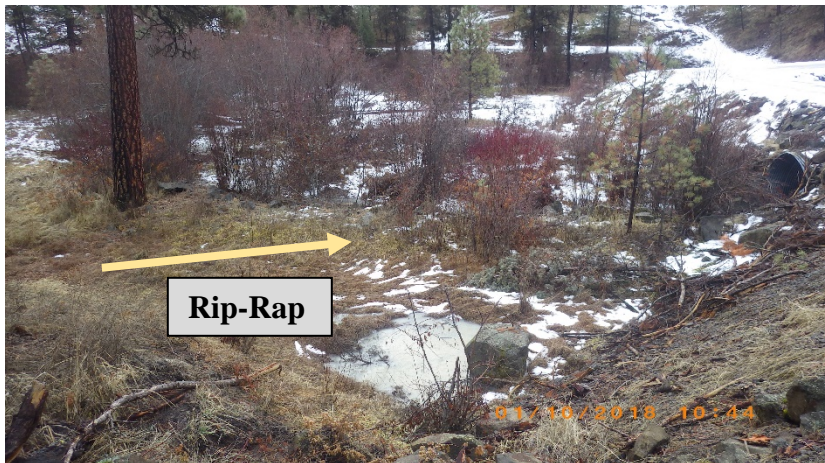
Figure 2. East Fork Beech Creek existing culvert inlet on National Forest System Road 3200935 showing rock rip-rap upstream and misalignment with valley bottom of culvert
