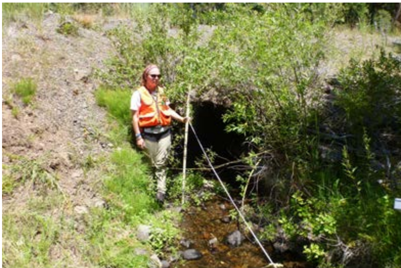
Figure 5. Tinker Creek existing culvert outlet on National Forest System Road 3600 showing perched outfall, no jump pool for fish passage, and streambed scouring from stream flow concentrated by undersized culvert
