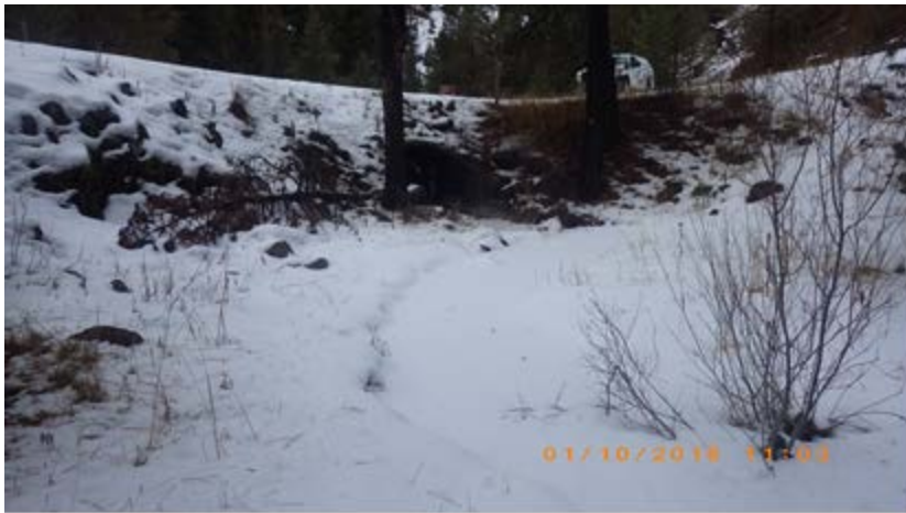
Figure 4. Tinker Creek existing culvert inlet on National Forest System Road 3600 showing large sediment wedge upstream of culvert and misalignment of pipe
