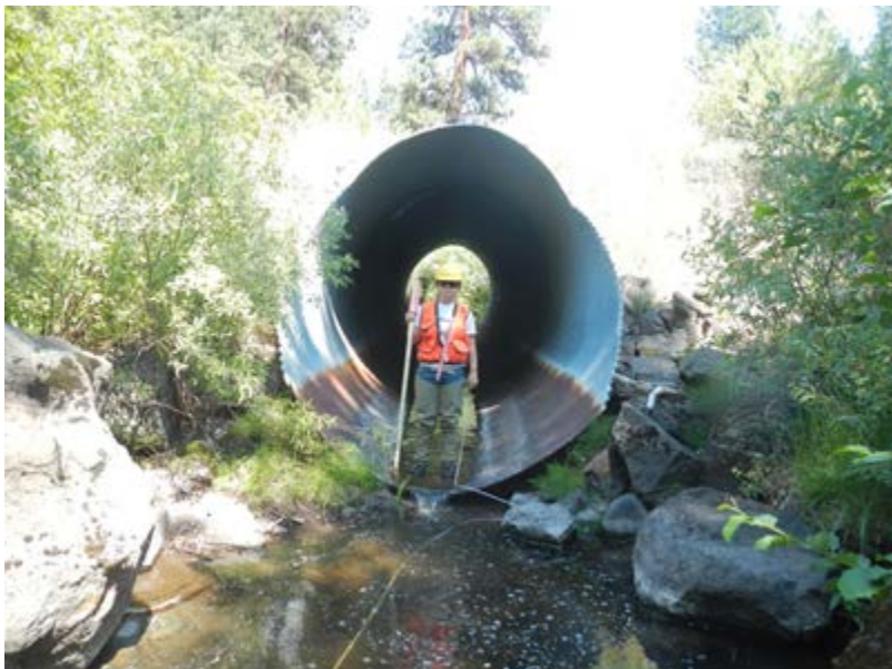
Figure 3. East Fork Beech Creek existing culvert outlet on National Forest System Road 3200935 showing large scour pool formed by excessive stream energy concentrated by undersized and misaligned culvert
