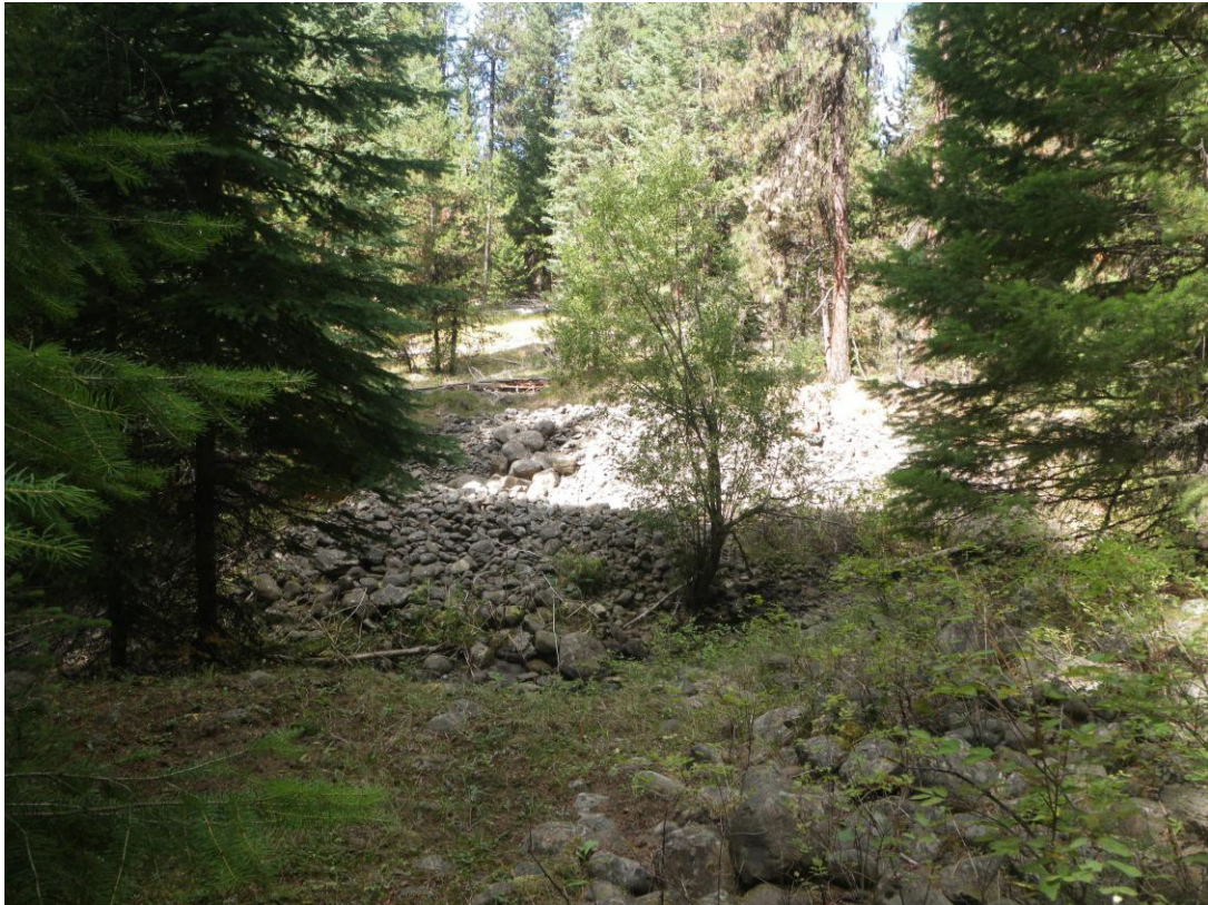
Mine tailing waste on historic floodplain Big Creek Reach 4
