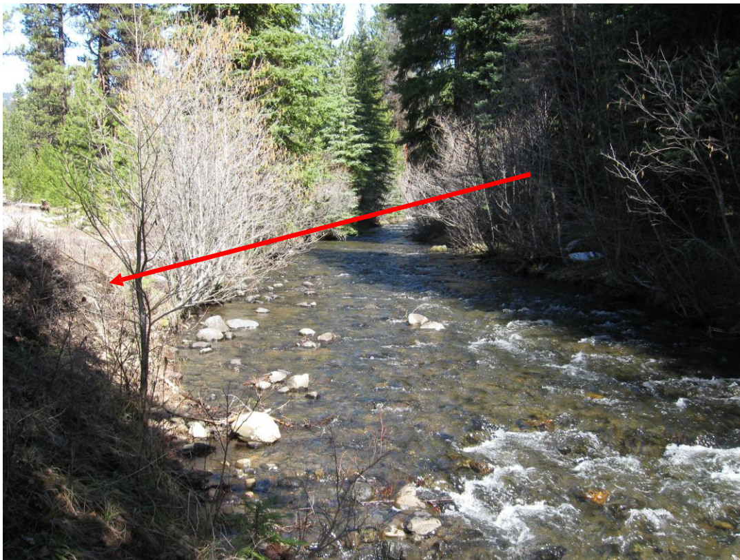
Mine tailing levee river left (Northside) Big Creek Reach 4
