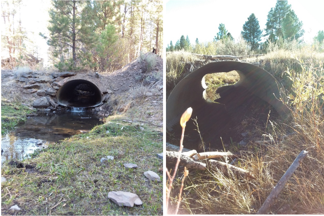
Figure 1: Left Photo - Forest Service road 1705954 at RM 0.1 of the closed road section is a seasonal fish passage barrier with large debris located at its inlet. Right Photo – Forest Service road 1705954 at RM 0.45 is undersized and is internally damaged with very little top fill present.
