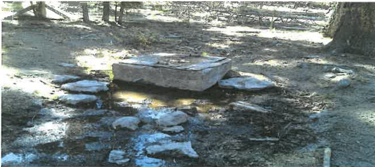
N 44.08432° W118.66142° spring source concrete head box.
