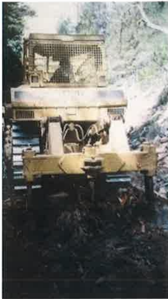
A grader outfitted with a ripper will be used to restore and re-contour the road prism where needed
