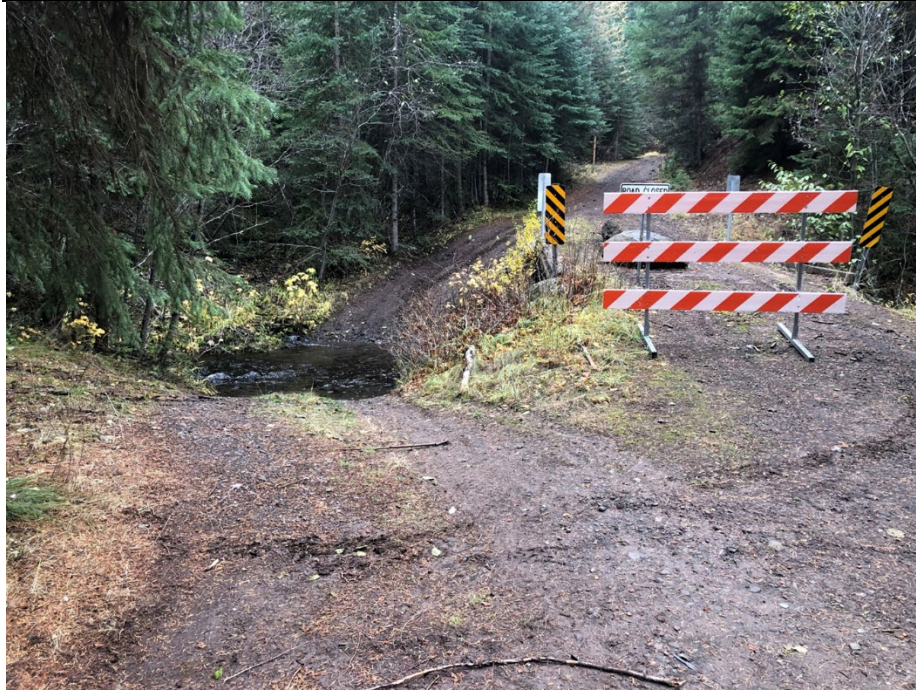
Figure 7. Bogue Gulch Bridge, user-created ford upstream of failed bridge.
