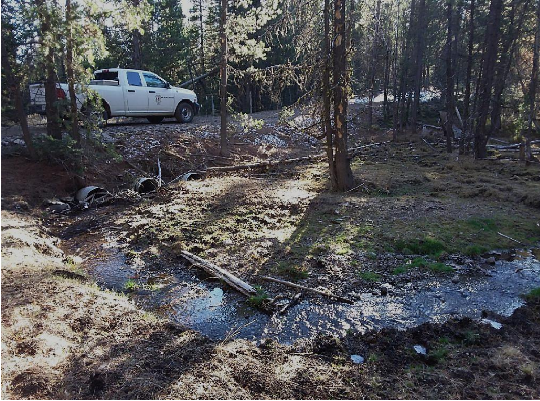
Figure 3: Upstream end of triple-barrel culvert crossing of Little Crane Creek on FSR 1660-478. Note the culverts are sunken/filling with sediment, also note substantial gravel bar that has developed above the crossing,
