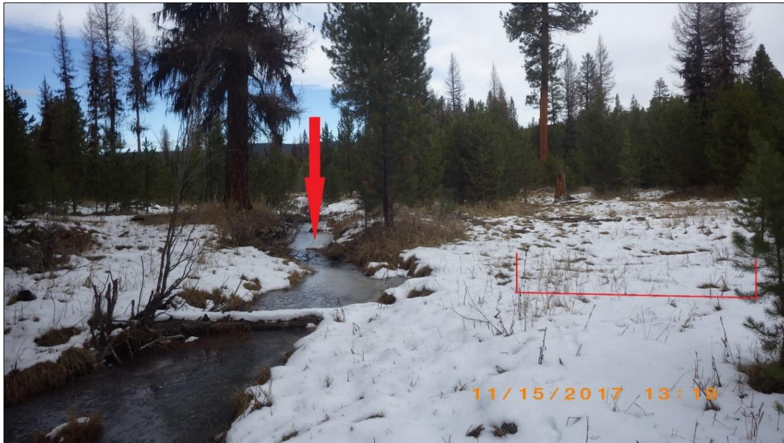
Figure 5. Location of proposed headgate and fish screen (red arrow) approximately 150 feet upstream of current diversion. Stream flow will be directed into historical flow path shown on right of photo (red bracket) and existing channel will be partially filled to convert into a ditch.
