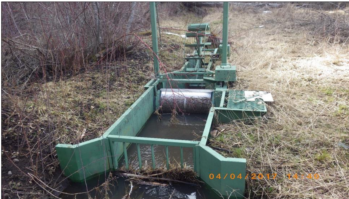
Figure 4. A rotary drum fish screen with water measuring device and headgate installed on East Fork Beech Creek. A similar design is proposed for the Marchbanks diversion on Wiwaanaytt Creek.
