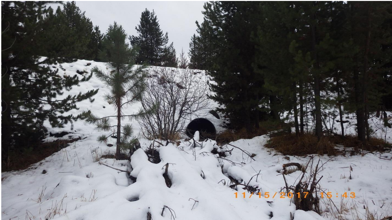
Figure 3: Existing culvert on FSR 2645-104 facing upstream. Stream channel is obscured by woody debris.
