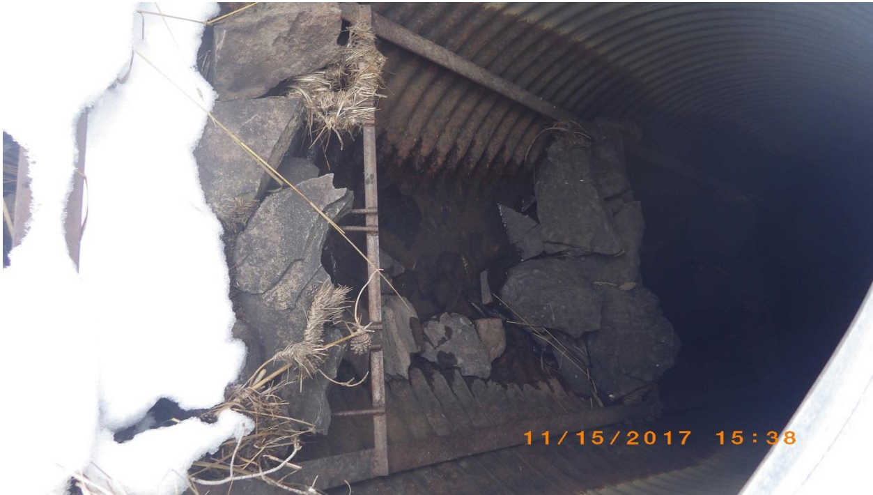
Figure 5: Inlet of existing culvert on FSR 2645-104 showing rock and steel baffles inside pipe.
