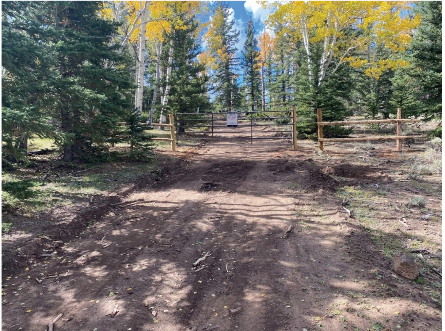
DANISH MEADOW ROAD - $108,000 Six miles of road was roto-milled and graded with appropriate water drainage. Before this project was completed, the only access to Danish Meadow was by All-Terrain Vehicles (ATV's) or horse back. Now it is passable with a two-wheel drive vehicle.
