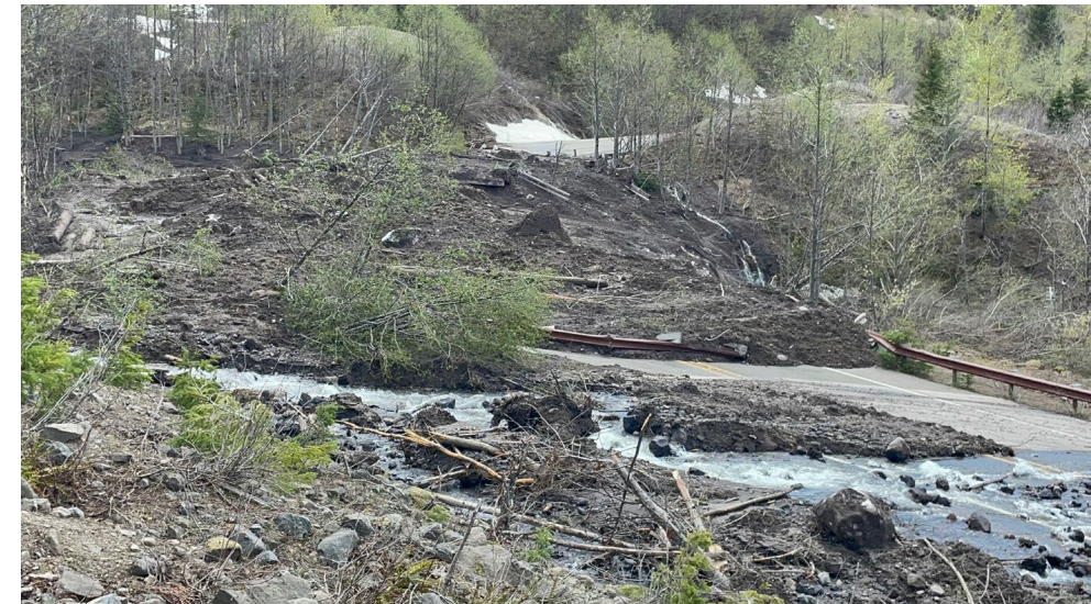
SR 504 Damage (Photo Credit WSDOT)
