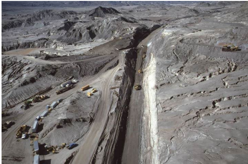
The Truman Trail (center) during operation of the pumping pipeline in the early 1980s
