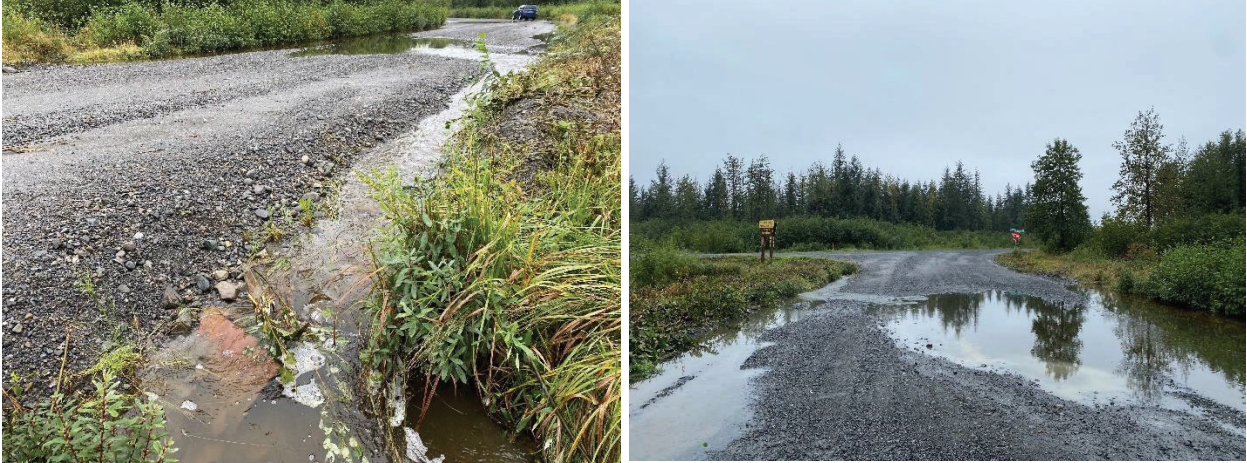
Figure 2: SHER 3 outlet (Left) – Culvert is not functional and water is being conveyed across road (Right).
