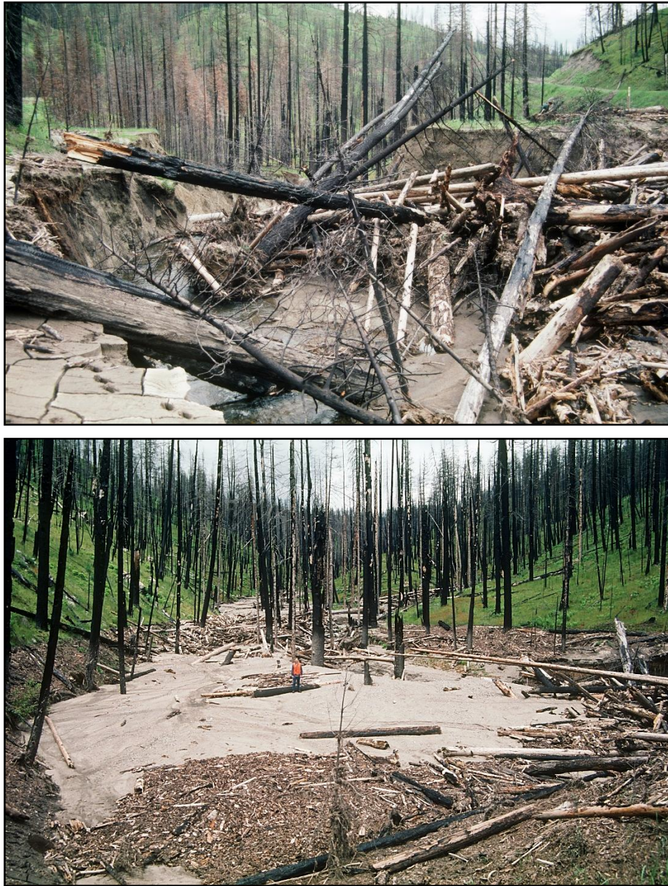
Figure 82 – Results of a debris torrent episode following a thunderstorm event in May 1988. Upper image shows aftereffects of a debris torrent spawned by an intense thunderstorm in May 1988. Not only did a debris torrent wash out the road, but it also inundated much of the floodplain, depositing large amounts of coarse woody debris and soil moved from adjacent uplands down to a floodplain.
