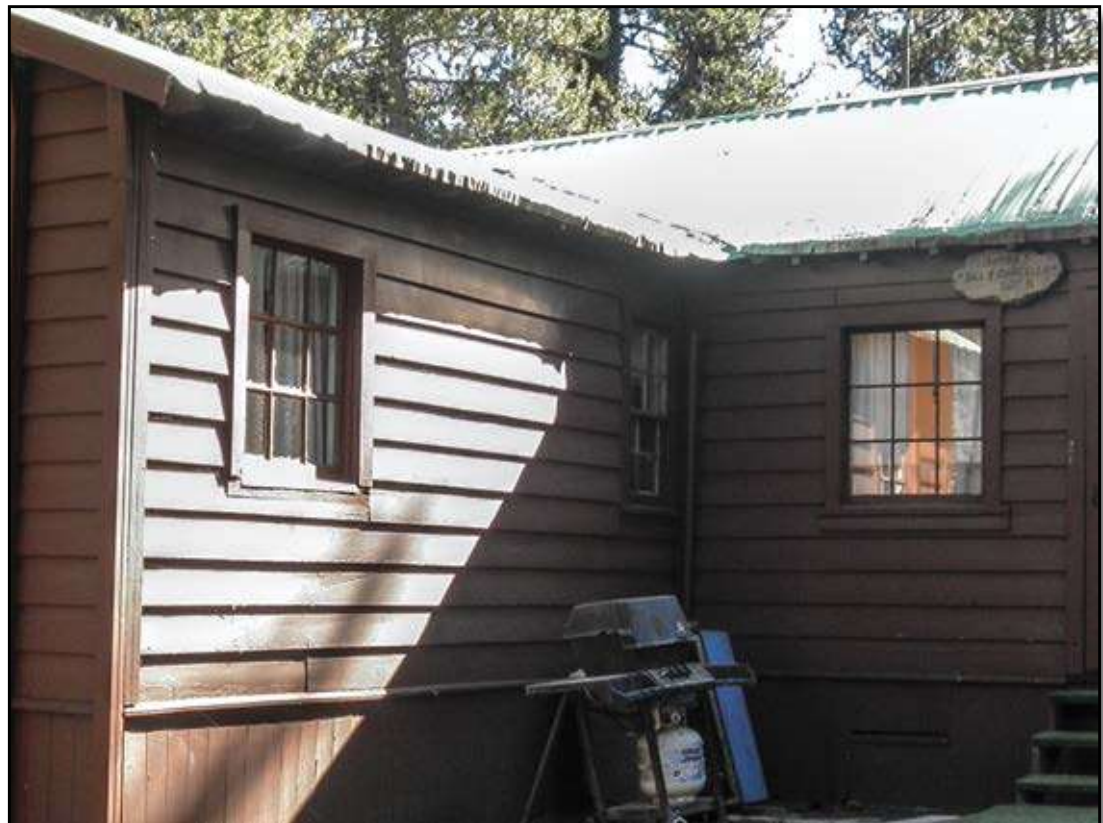
Figure 5—Part of the windowsill broke off of this recreation residence's left window. Replacing it with a windowsill that exactly matches the other windows is routine maintenance.
