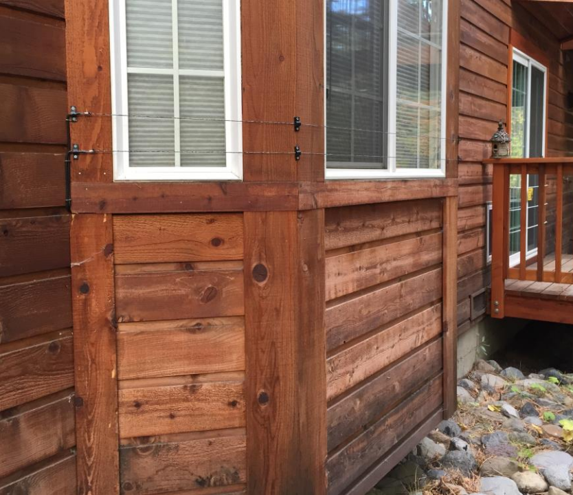
Electric fencing along windows
