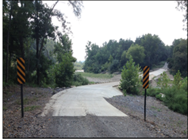
Extended Concrete Approaches with Slope Paving to Reduce Erosion at the 53000 Glover Bridge
