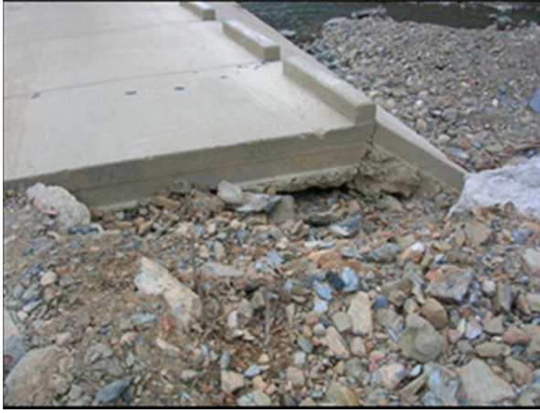
53000 Glover Bridge Washed Out Approach
