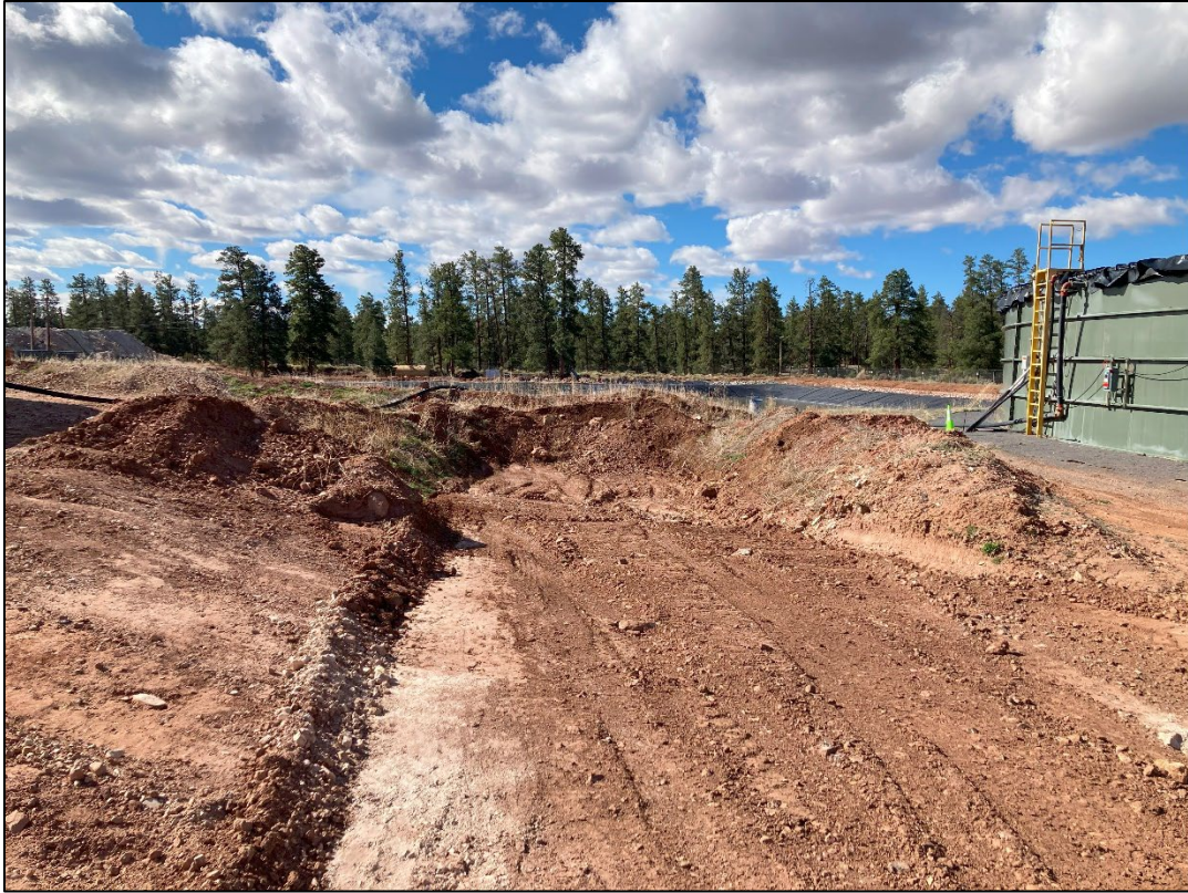
Photo 7 – Rainwater catchment (empty) between the two water tanks in NW perimeter. (Apr. 29)
