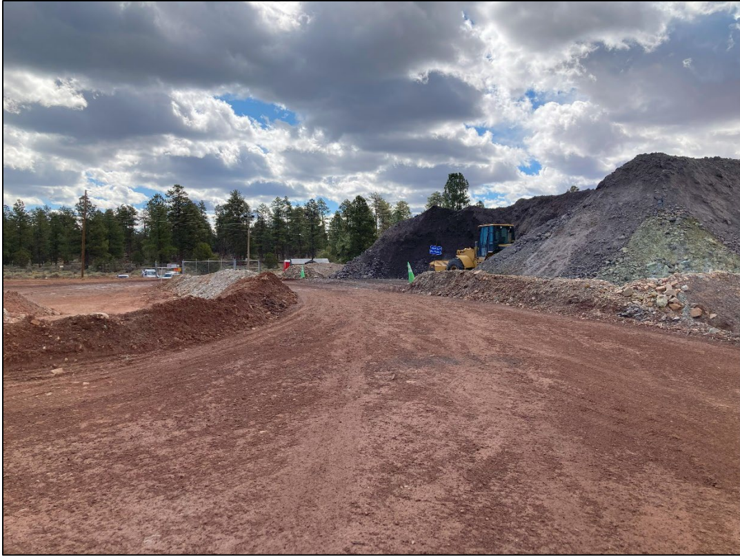
Photo 23 – Overlooking the ramp used by haul trucks to access the ore pad. (Apr. 29)
