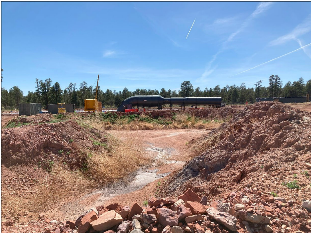
Photo 10 – Central rainwater catchment. (May 23)
