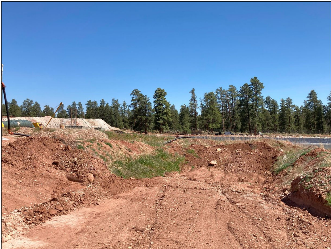
Photo 8 – Additional look at rainwater catchment (empty) between the two water tanks in NW perimeter. (May 23)
