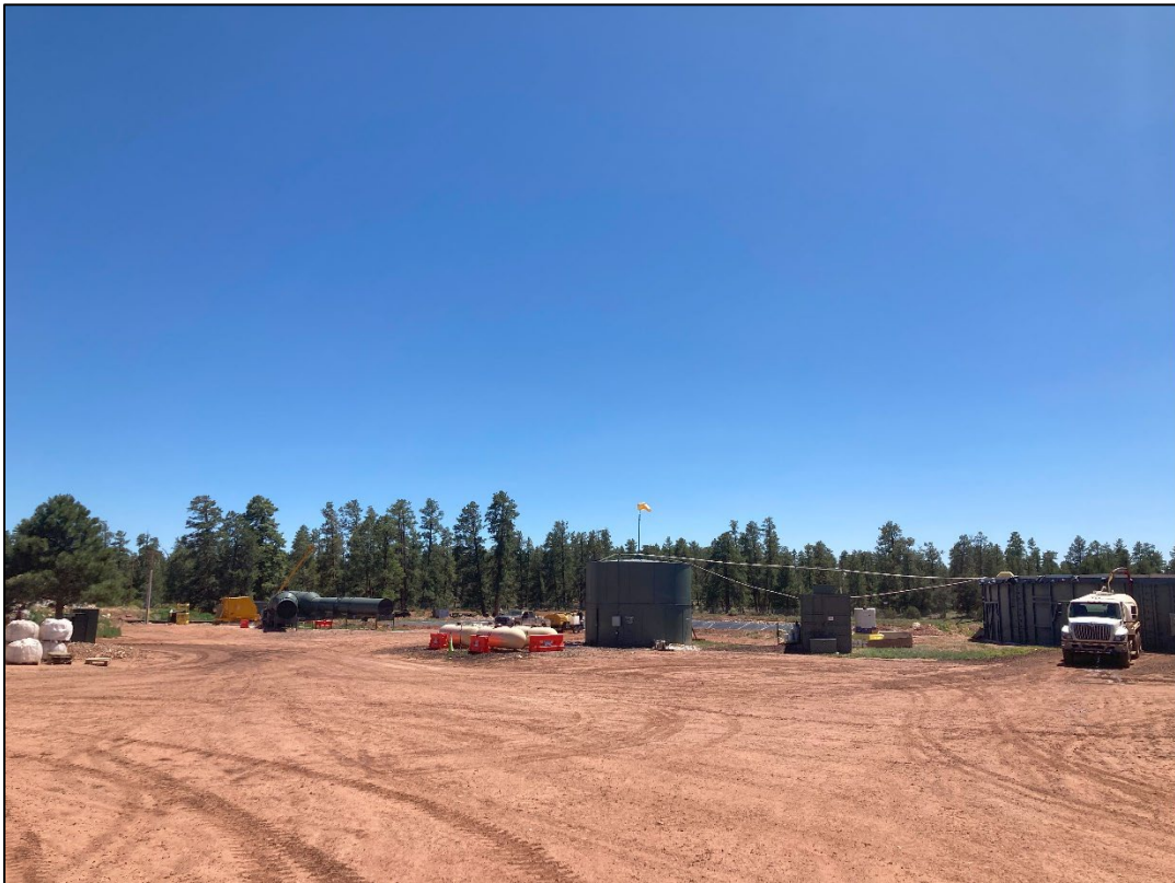
Photo 6 – Additional view of the propane and water storage tanks. (Jun. 23)
