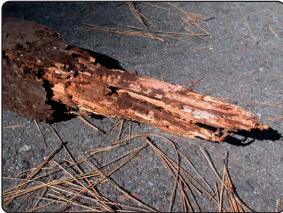
Figure 180. Damage to sign post caused by termites.
