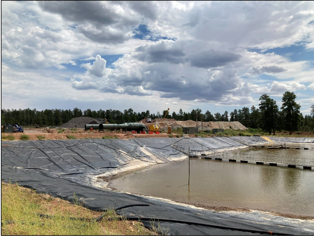
Photo 11 – Non-stormwater impoundment with ventilation system in background. (Aug. 22)
