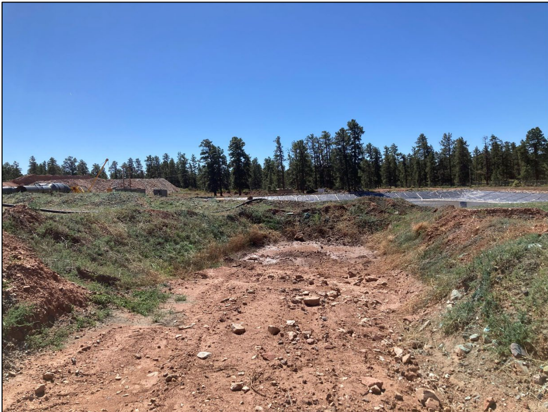
Photo 8 – Weeds near rainwater catchment removed, with minimal moisture within the catchment in September.
