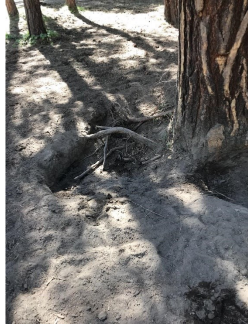
Figure 36: Holes and tree root damage caused by wild horses at a dispersed recreation site in the Territory.
