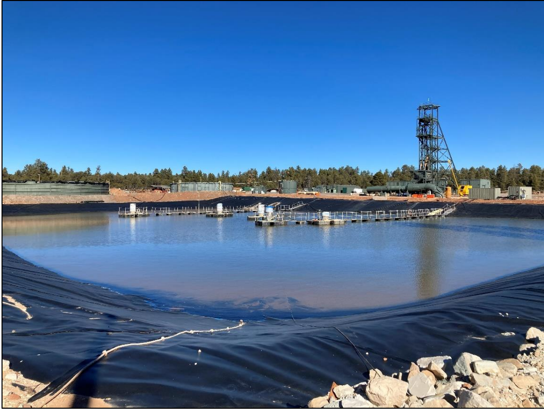
Photo 13 – Non-stormwater impoundment, facing NE. All evaporators were offline. (Dec. 17)
