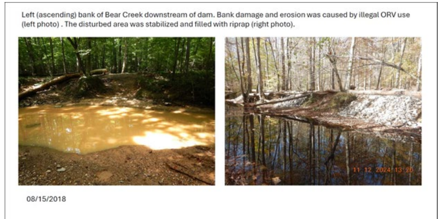
Figure 8. Bear Creek Erosion Control Project before and after treatment. Credit John Moran
