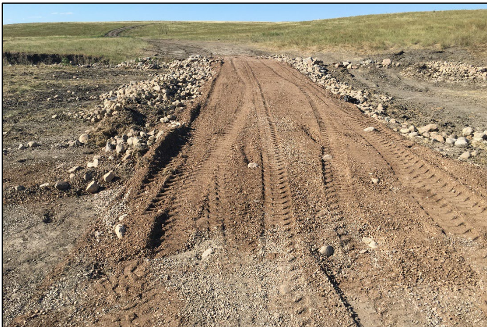
Figure 41. Culvert, rock, gravel, and coarse aggregate material used as a replacement for failed geofabric fabrics. Forest Service Road #253, Fort Pierre Geographic Area. Photo July 2020 by Dan Svingen.
