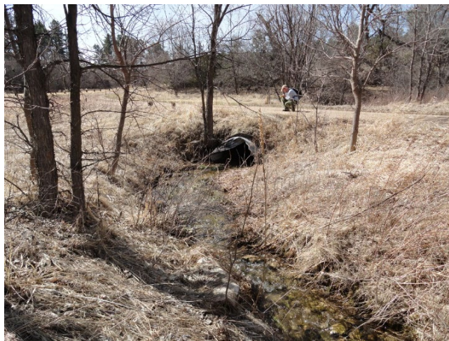
Photo: 11. Before: an undersized culvert was starting to collapse and was a barrier for aquatic organism passage and high flows.
