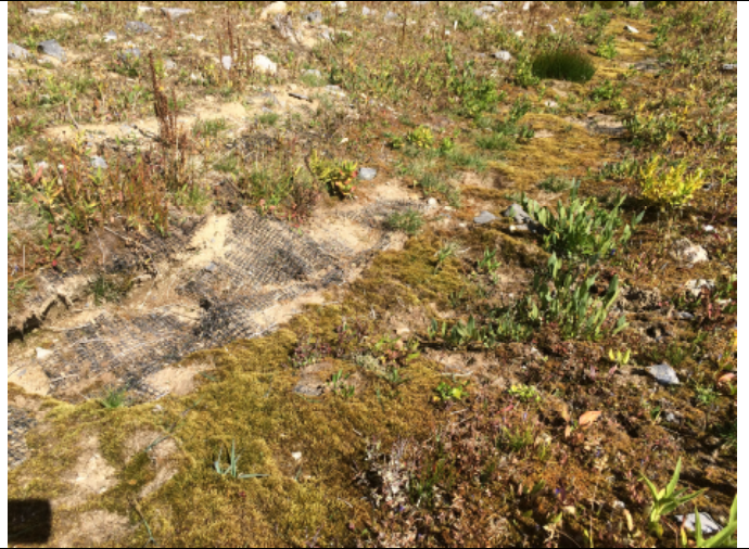
PHOTOGRAPH 2 View of failed vegetation mats
