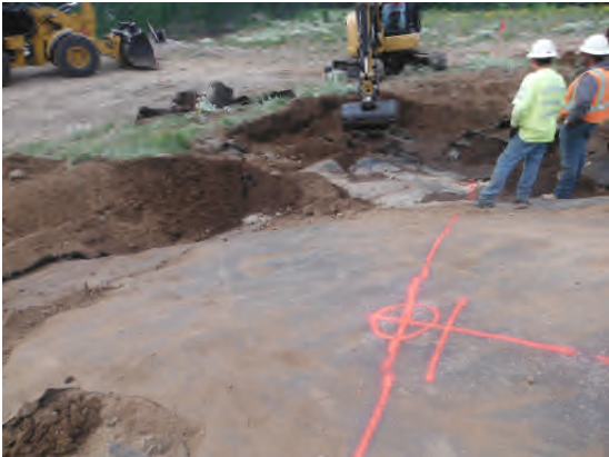
Excavating toward road to west of repository. "X" marks future location of sump access tube.
