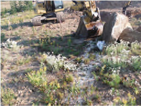
Absorbent materials on ground to control hydraulic fluid spill.
