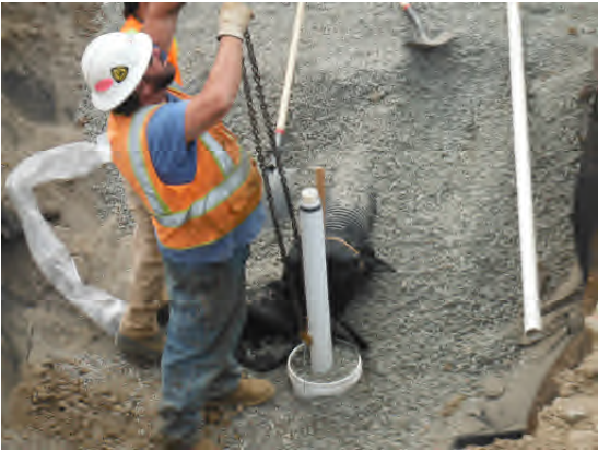
Installing sump access tube. Buckets are used to protect tube during compaction of backfill.
