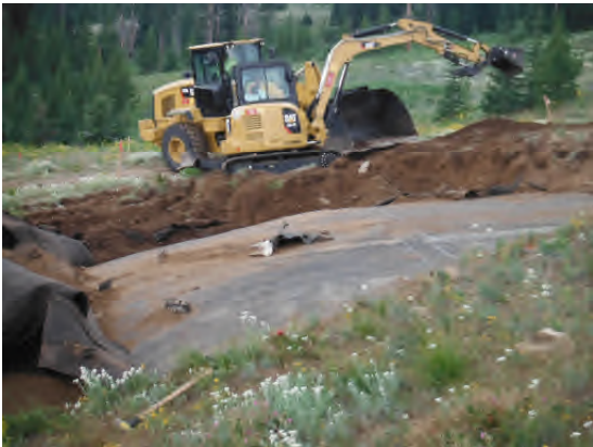
Geocomposite/HDPE liner exposed in excavation. Holes visible at left (south) side believed to be present prior to excavation. Note lack of sand layer between layers of synthetic liner.
