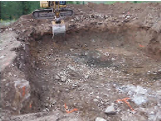
Final gallery excavation. Orange lines mark top of gravel subgrade and pipe junctions.
