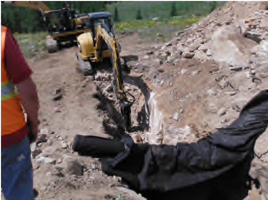
Breaking rock with malfunctioning hammer.
