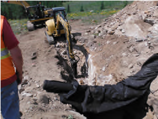
Breaking rock with malfunctioning hammer.
