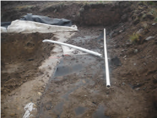
Sump access tube solid and slotted 2" pvc.
