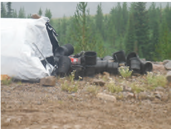
Drain pipe couplings, gaskets, cement.
