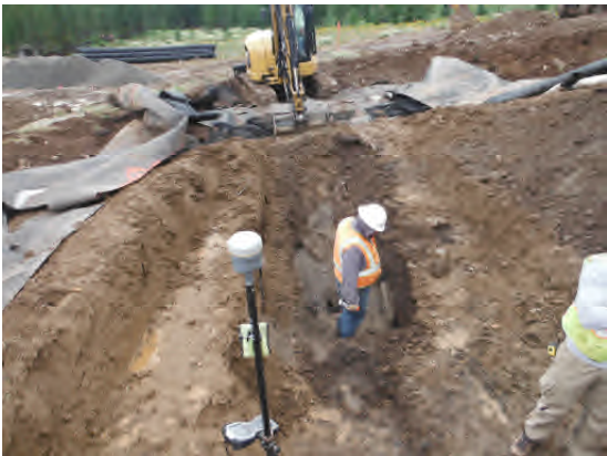
Excavating bottom liner. Rocks to right of worker were pulled from lower portion of drainage gravel.
