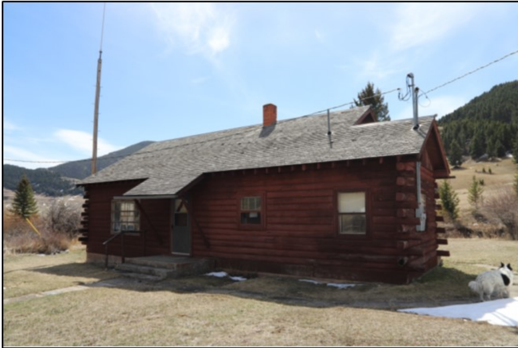
MT_StillwaterCounty_MeyersCreekWorkCenter_0014. Exterior view of the Feature 2 residence, May 19, 2022, View to southeast. (Photographer: Tim Urbaniak)
