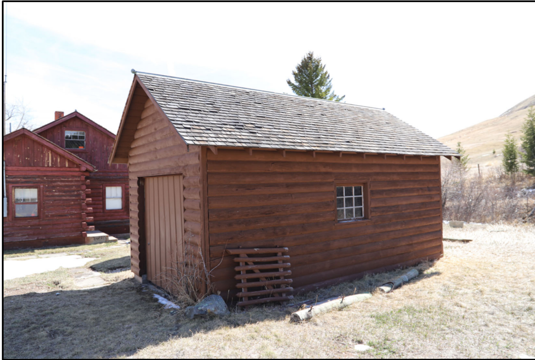
MT_StillwaterCounty_MeyersCreekWorkCenter_0016. Exterior view of the Feature 3 garage, May 19, 2022, View to east. (Photographer: Tim Urbaniak)
