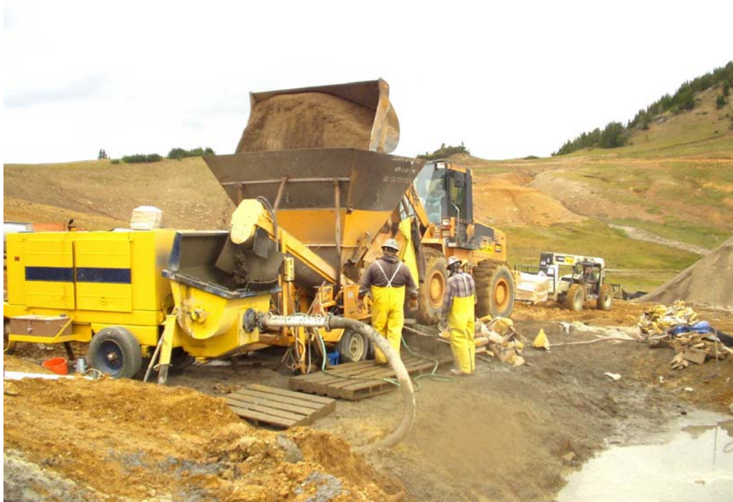
Figure 20. Continuous 15 Cubic Meter/Hour Concrete Batch Plant at the Como Raise
