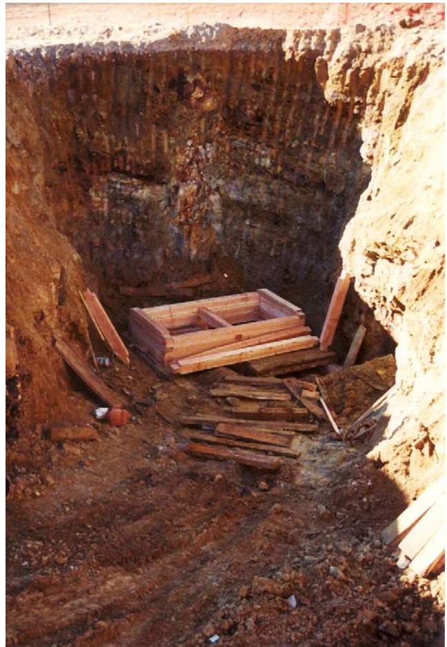
Figure 5. Como Raise Collar Showing Original Timber-Bearing Set, Raise Collar Cribbing, and Excavation
