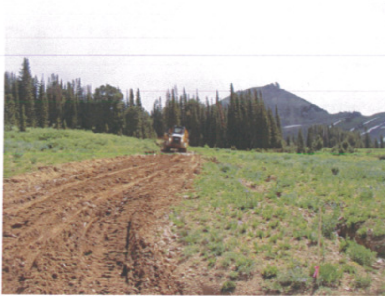
Photograph 8 – Unstable Sub-Grade along the Lake Abundance Road
