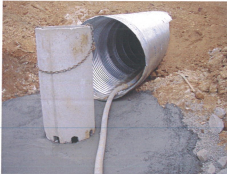
Photograph 3 – Riser and Concrete Pad – McLaren Adit Water Collection System
