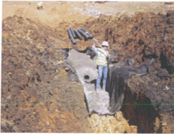
Photograph 4 – McLaren Adit Water Discharge Line
