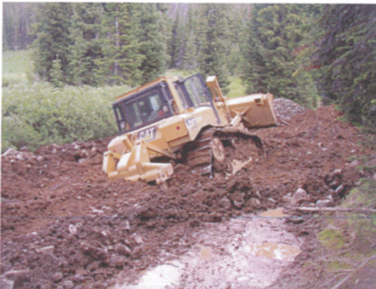
Photograph 7 – Unstable Road Subgrade (Lake Abundance Road)
