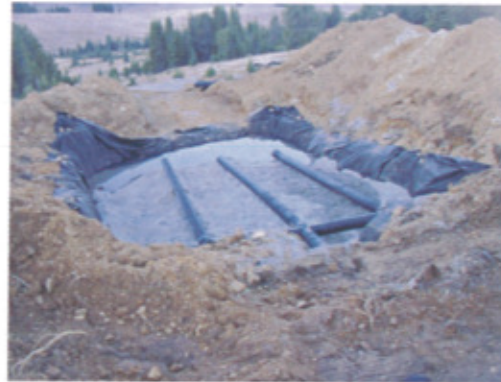
Photograph 5 – McLaren Adit Infiltration Gallery
