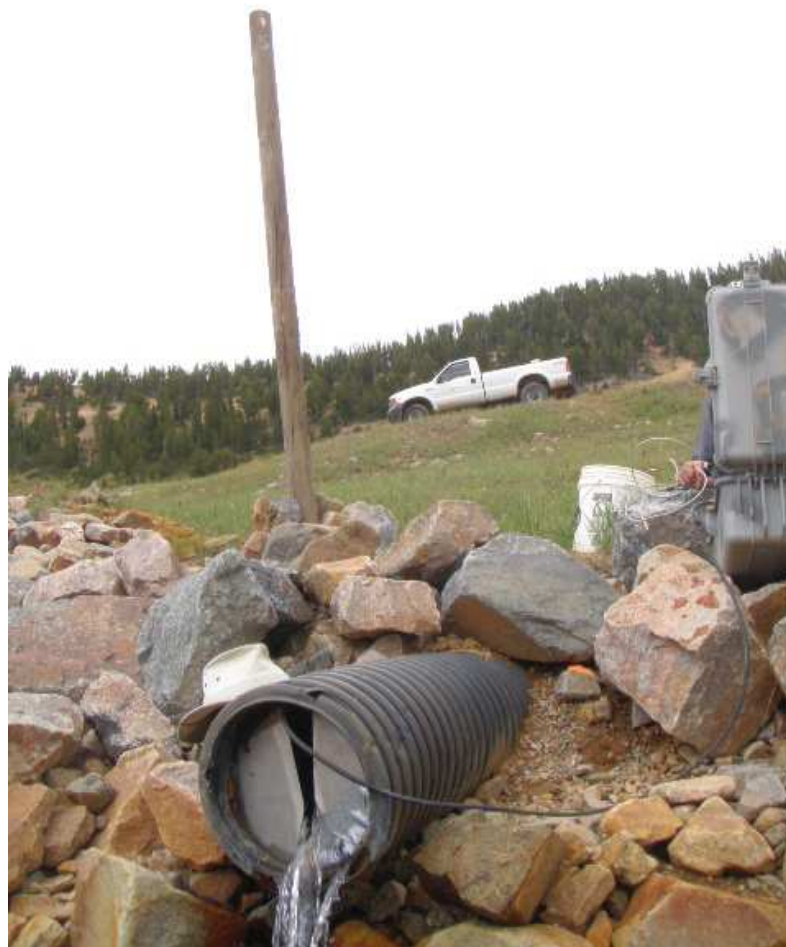
Figure 3. McLaren Pit subsurface drain DCSW-101.
