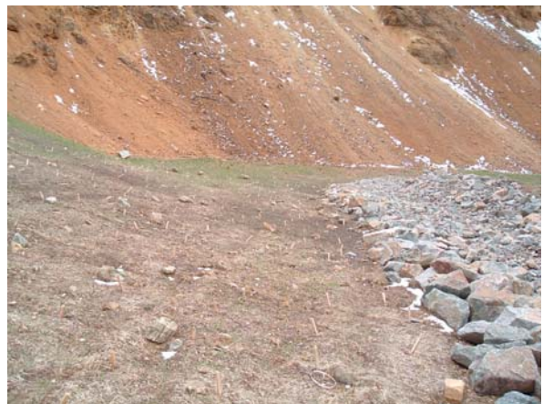
McLaren Pit Cover – Low Cover at Base of Highwall 2004 Reclamation Monitoring
