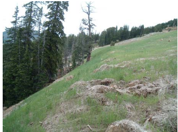
McLaren Pit Cover – Soil Slump Above Toe Berm 2004 Reclamation Monitoring
