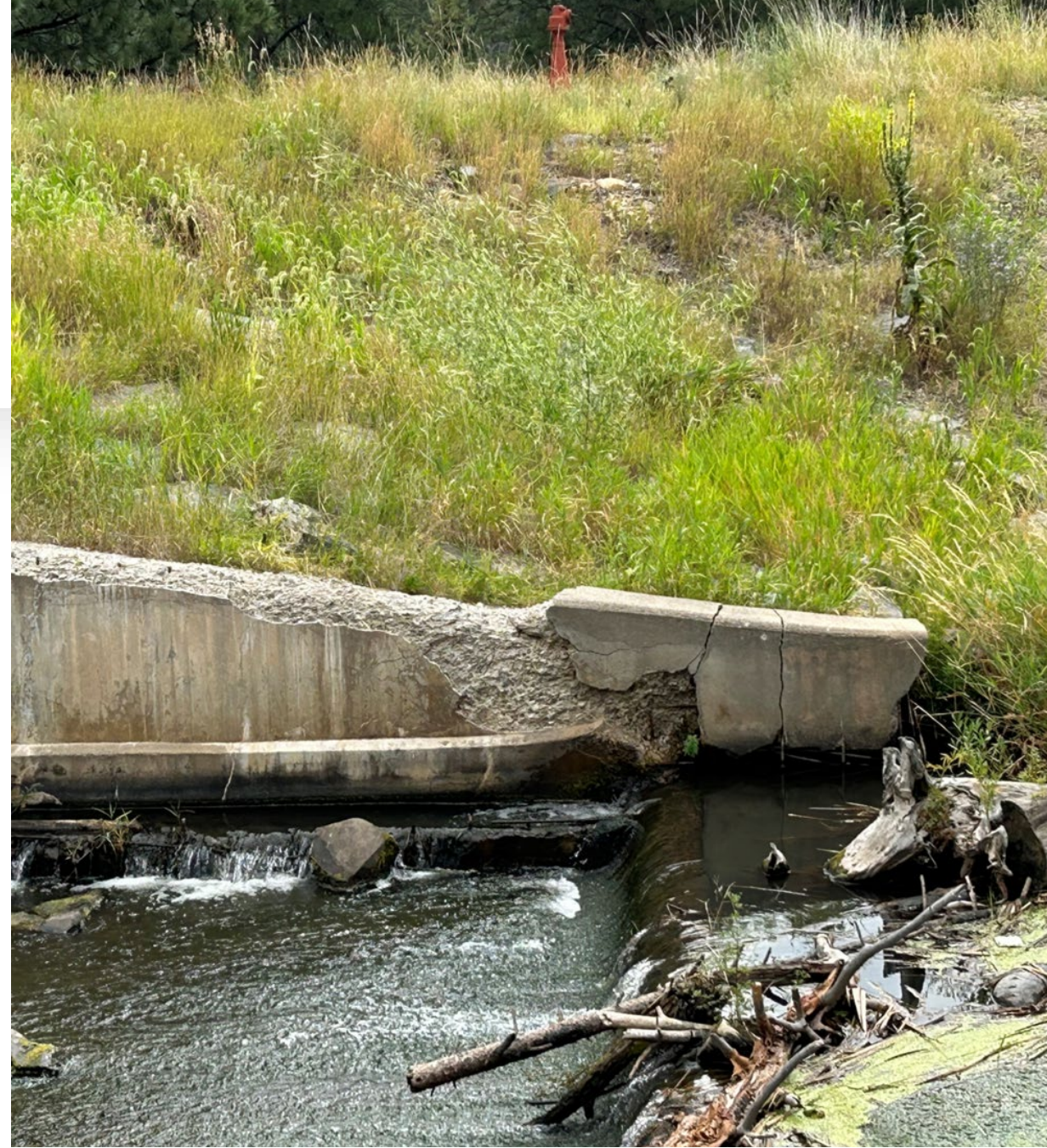
Image: spillway entrance right wall – deteriorating concrete, end of the wall is breaking off vegetation growing, debris blocking the entrance.
