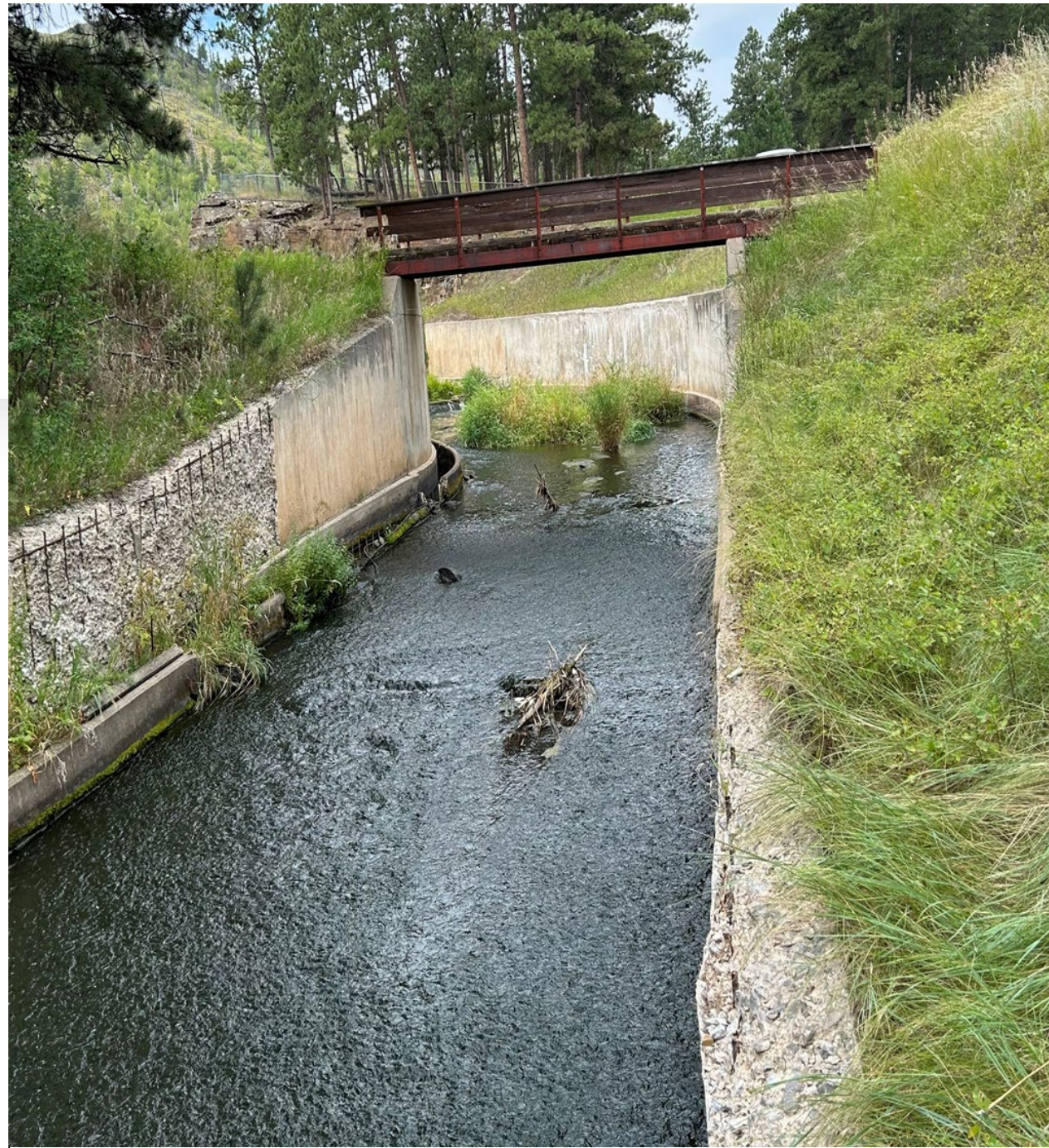
Image: spillway – deteriorating concrete, rebar exposed, vegetation growing, debris in the spillway.
