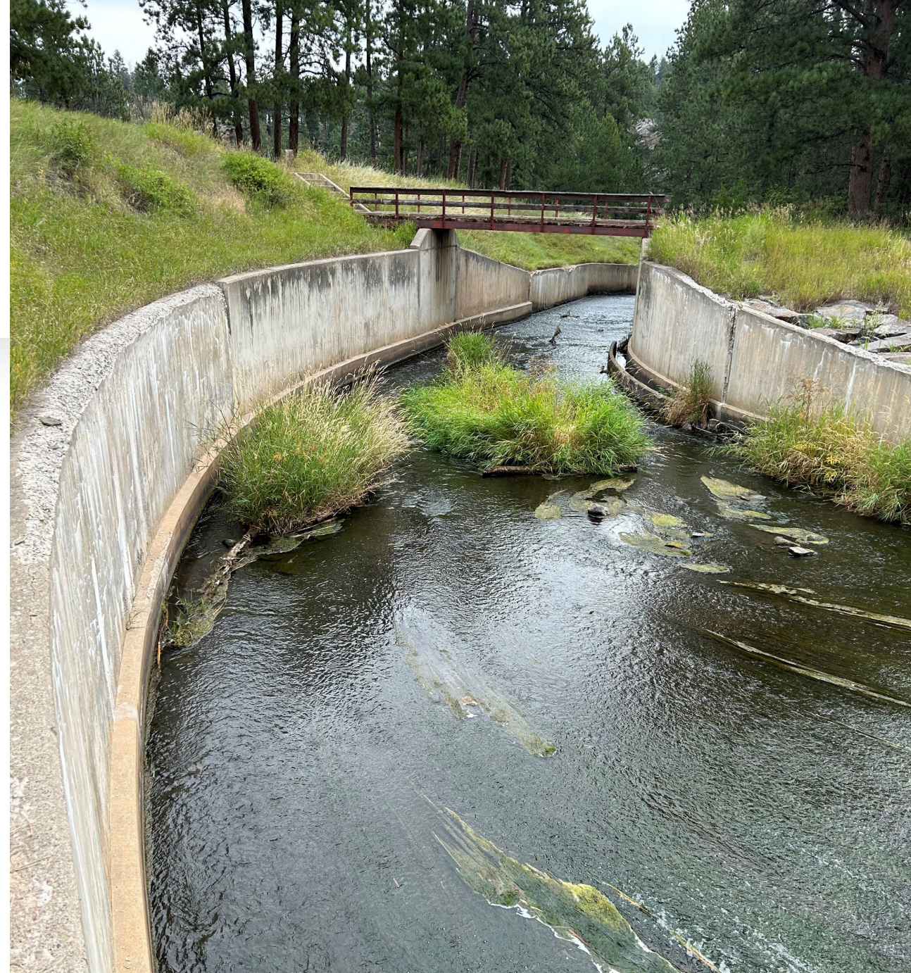
Image: spillway entrance – deteriorating concrete, vegetation growing, debris blocking the entrance.
