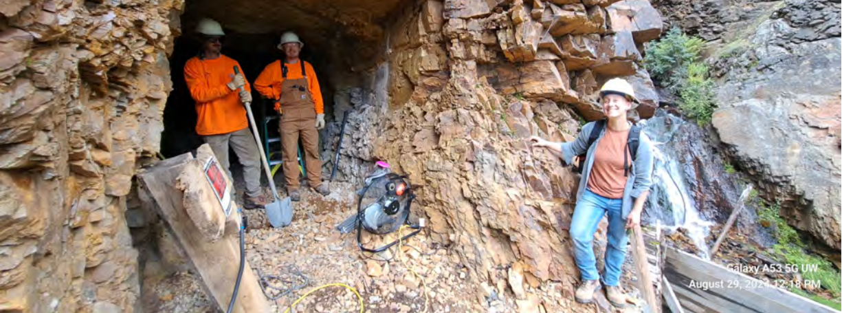
Emma Reinemann stands at one of the mine openings slated to be closed.
