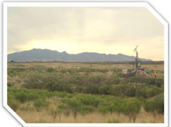
Drilling boreholes on Bella Vista led to the identification of the ideal recharge site on Coyote Wash. Photo taken by Brooke Bushman.
