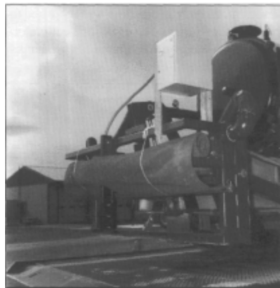
Figure 3. The initial steam injection system used an undercutter blade. Steam was vented from the back of the blade.
