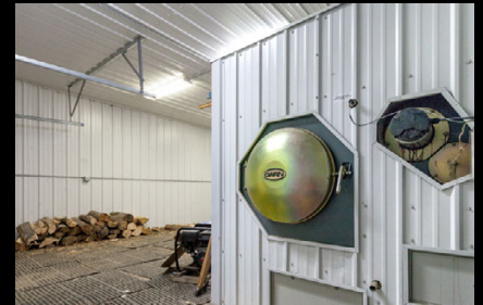
Biomass Heating Plant
