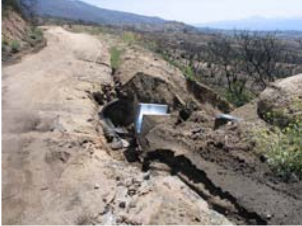
Fig. 2.37. Failure of overside drain at mile point 1.4 on Anderson Truck Trail. Photo taken on Apr 7, 2004.
