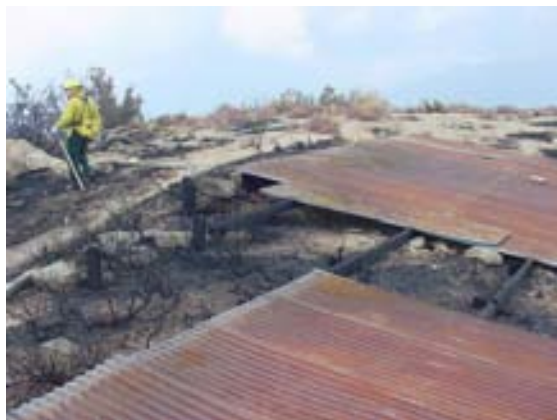
Fig. 5.1. Burned components of the Sunset Peak Lookout site, looking southwest. Site visited in November following fire.
