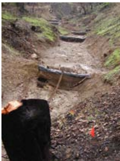
Fig. 4.16. Water flowing under structure in foreground and sediment overtopping and going around structure.
