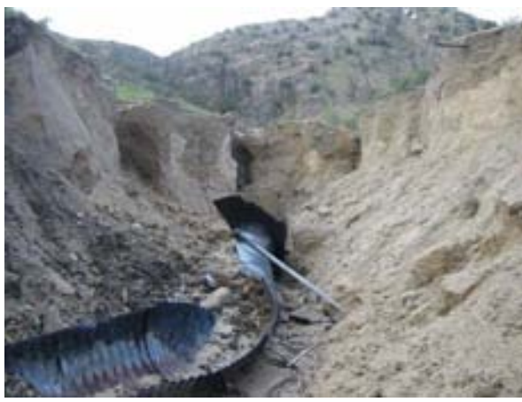
Fig. 3.62. Failure of rolling dip and upside drain along Big Tree Cucamonga #1N34. This occurred following October, 2004 storm events. Treatment was planned here but not completed before the October, 2004 rain events. Milepoint was unknown.
