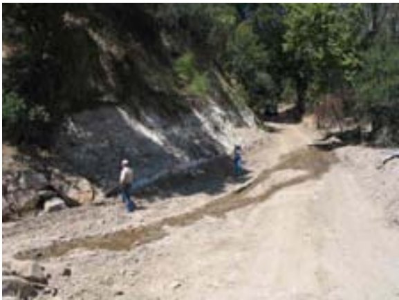
Fig. 4.27. Further erosion and 3-4 ft of new sediment
