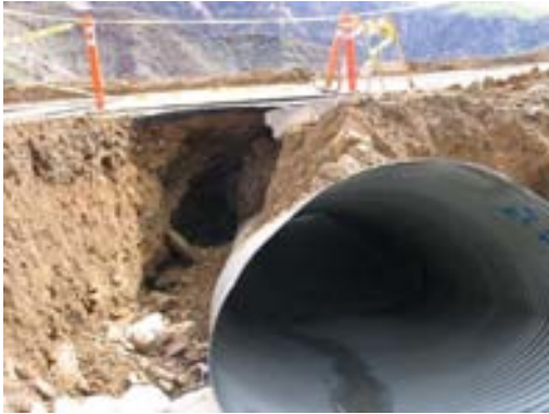
Fig. 4.31. Culvert that has failed located at mile point 0.4 on Squaw Flat Rd.
