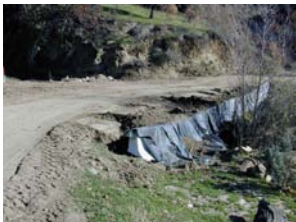
Fig. 4.23. Low water crossing with K-rail covered with filter cloth (mile point 1.2).
