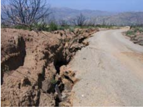
Fig. 2.35. Gully formed on side of Anderson Truck Road.
