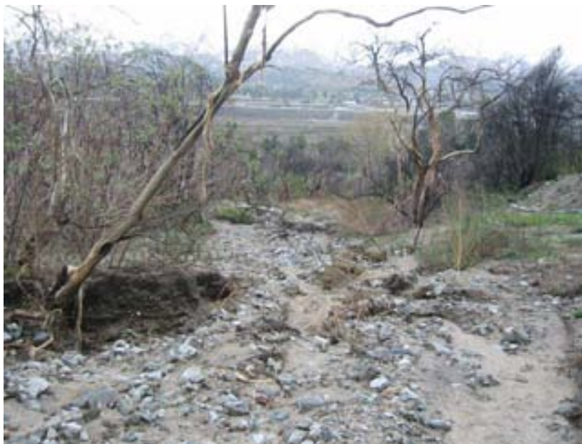
Fig. 3.58. Blowout of strawbale check dam located in lower channel (view looking down channel).
