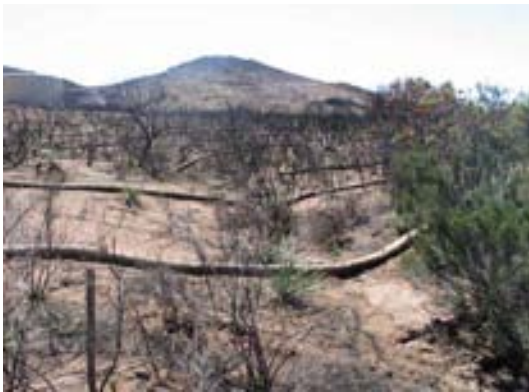
Fig. 2.24. Fiber rolls incorrectly placed across drainage.
