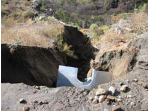
Fig. 2.39. Failure of upside drain at mile point 1.49. This failure occurred during the October, 2004 rain events.
