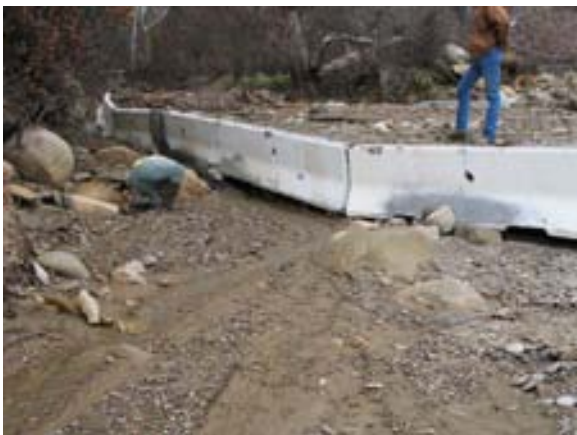
Fig. 4.26. Water worked itself around the K-rails.
