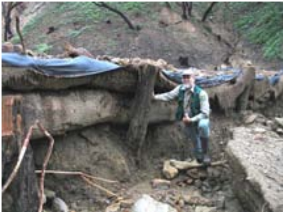
Fig. 4.19. View of log check dam being undercut. With the check dam filled to capacity with sediment, there is nothing reducing the energy of the water flow.
