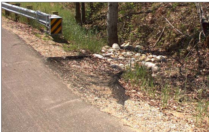
Lead out ditch with energy dissipater (Michigan)
