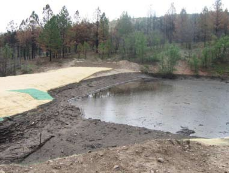
Upper retention dam after first thundershower following fire (notice spillway overflow).
