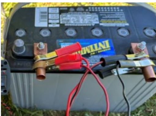
Figure 7 Battery with controller and inverter.
