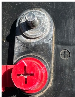
Figure 15 A battery terminal with corrosion.
