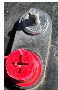
Figure 17 A clean battery terminal without corrosion.
