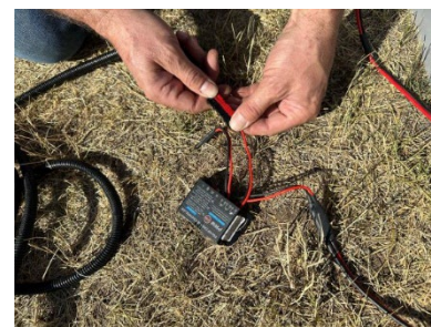
Figure 8 Solar panel connection to the controller.
