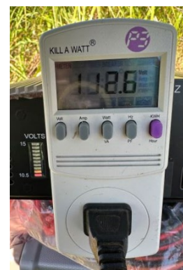
Figure 10 Here's the inverter output voltage (112.6 VAC) with a 1500 watt rated unit delivering 800 watts to a coffee pot (about 70 Amps). This is on the low end of the output voltage, but there is quite a bit of sag due to the high current voltage drop in the DC cables going to the inverter (3 SLAs in parallel for 12 Volts at roughly 300 AH capacity).
