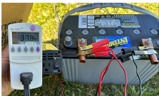
Figure 9 A battery hooked up to controller and inverter, being read by a voltmeter.
