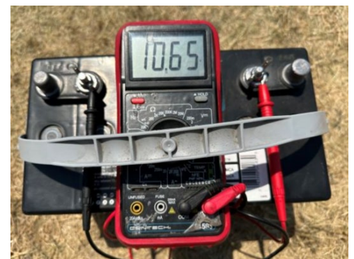
Figure 4 A battery that is fully discharged.
