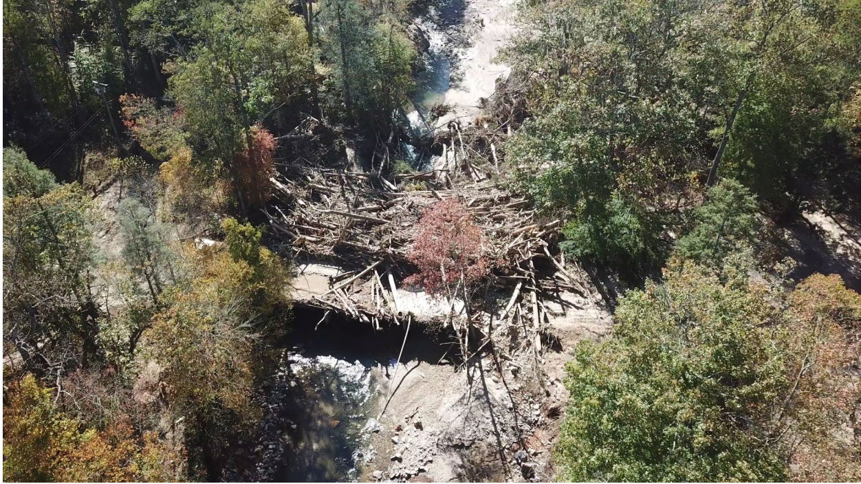
Figure 2.- Oblique image of a log jam affecting the Black Mountain Campground Bridge on the Pisgah NF.
